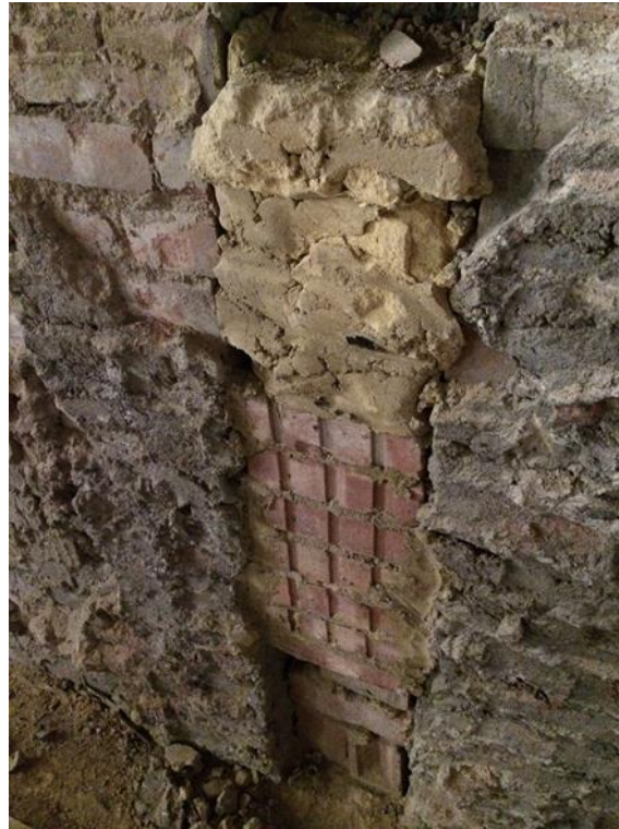
Figure 16. Close up of void Feature at second floor level (Walkden floor levels) of the RCGP (Mott MacDonald, 2019)
