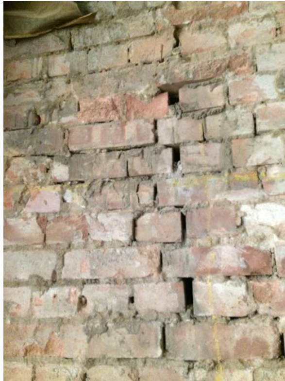
Figure 15. RCGP elevation at first floor (Walkden floor levels) showing brickwork needing repair (Mott MacDonald, 2019)
