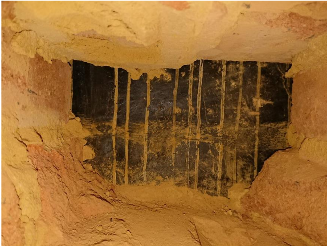
Figure 11 A 'window' in the basement party wall of Walkden House - brick infill removed revealing RCGP brick covered in bitumen (Mott Macdonald, 2019)
