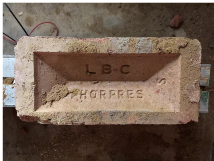
Figure 10 – Phorpres type brick with deep frog and stamp, found in the Walkden House Wall
