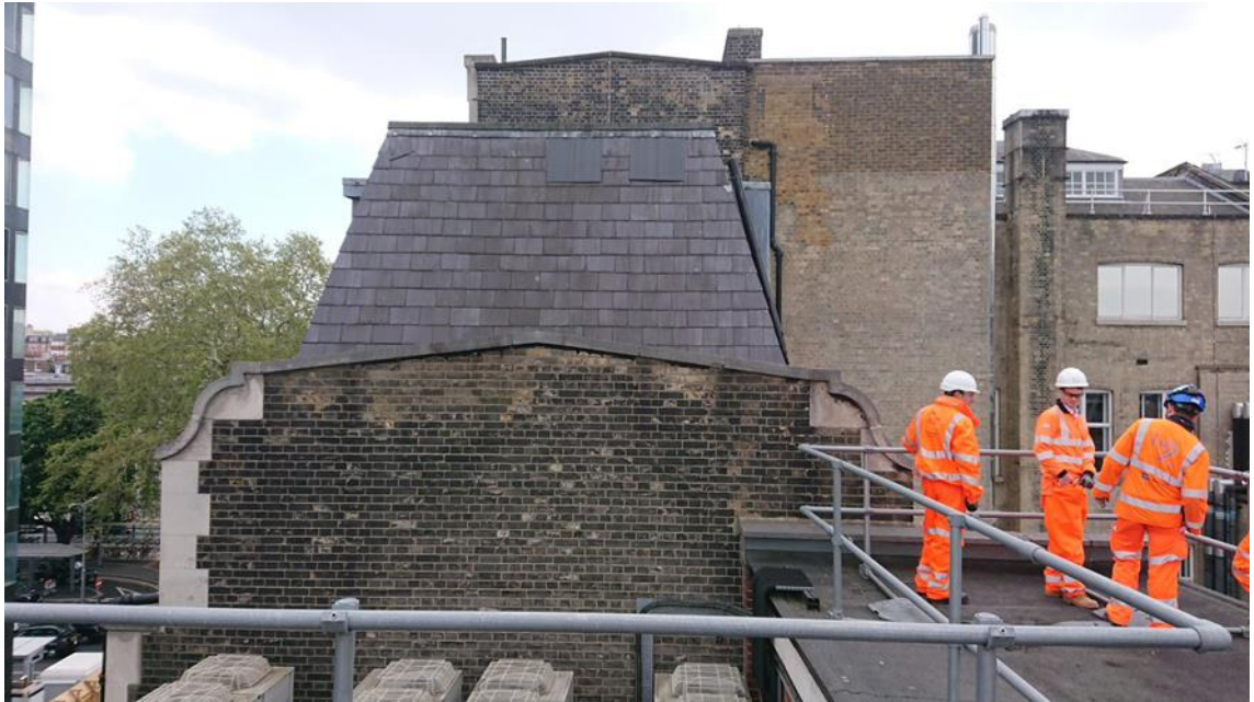
Figure 5. RCGP party wall with Walkden House, viewed from the north from the roof of Walkden House (Mott Macdonald, 2019)
