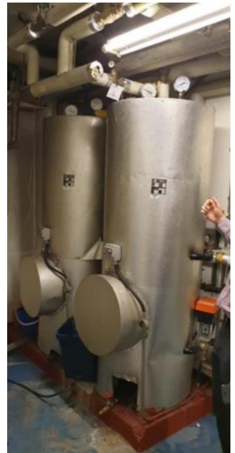
Figure 5 – Existing Cylinder Calorifiers
