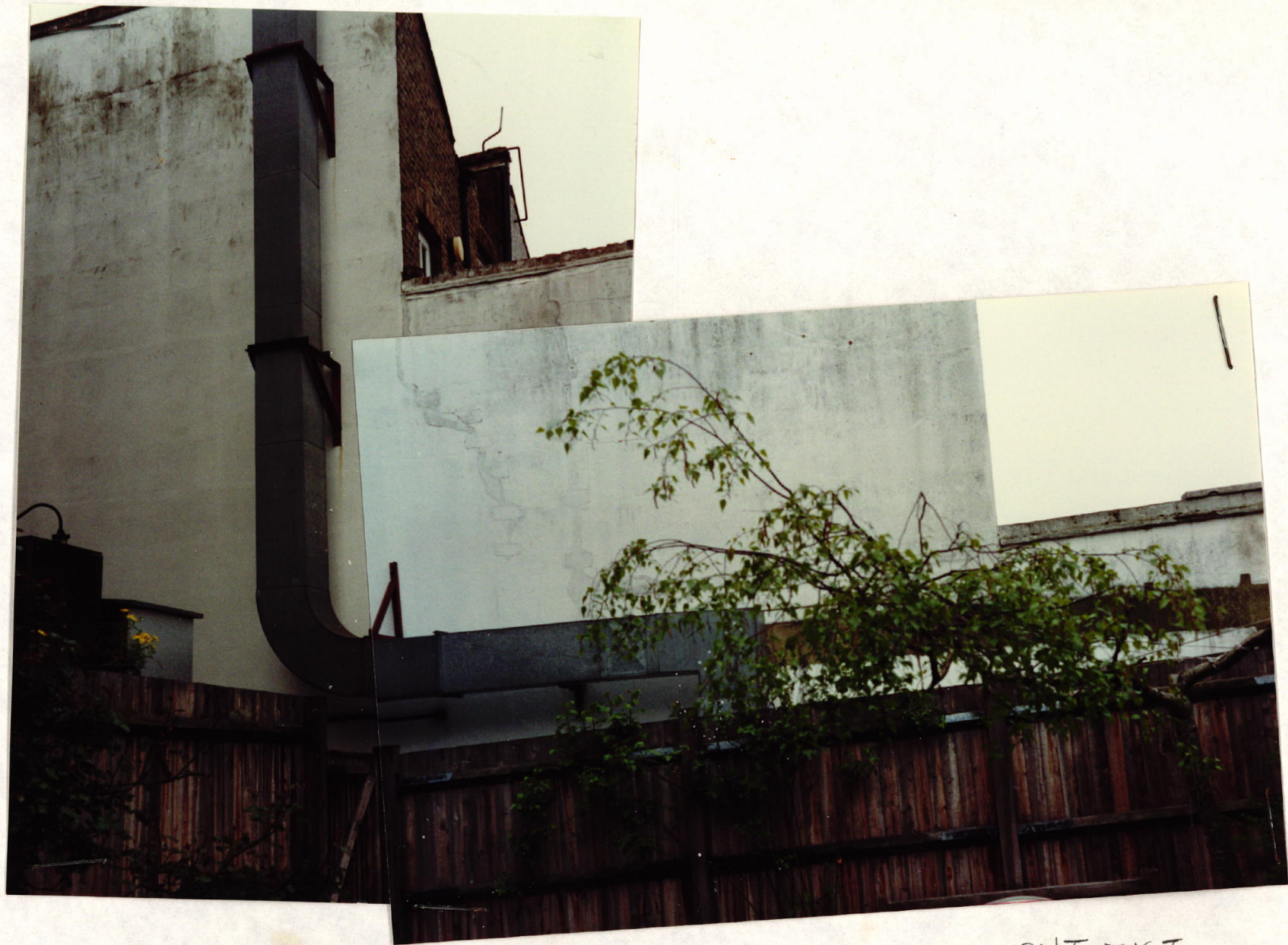
VIEW FROM PUB GARDEN AT REAR OF FLASK OF VENT DUCT FOR NO. 16 RESTAURANT (ON LIMITED PERIOD P.P.) - ON 16'S WALL - BUT OVERHANGING 14'S PROPERTY
