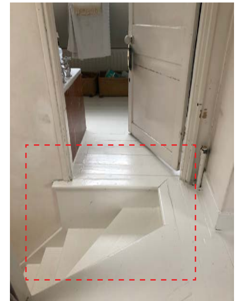
Dangerous north staircase
