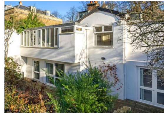
A photograph of the existing north end of the rear elevation shows little original historic fabric, and the insensitive massing of the 1960s extension which overlaps the historic transept.
