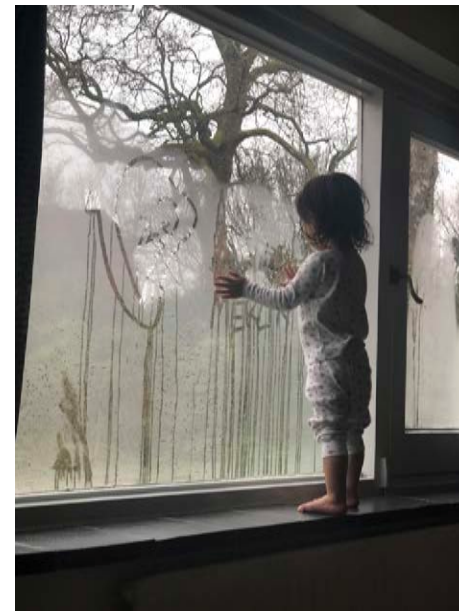
Poor quality construction of windows
