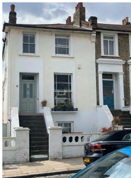
Original configuration of front windows to neighbouring building and original capped squat columns either side of entrance.
