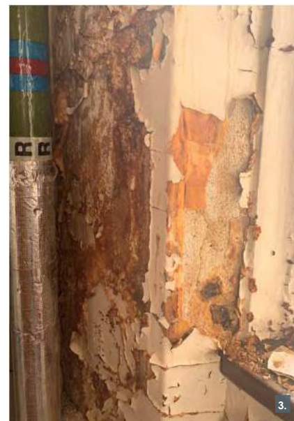
1- Plaster damage to window reveal (water ingress) 3- Plaster damage due to water ingress
