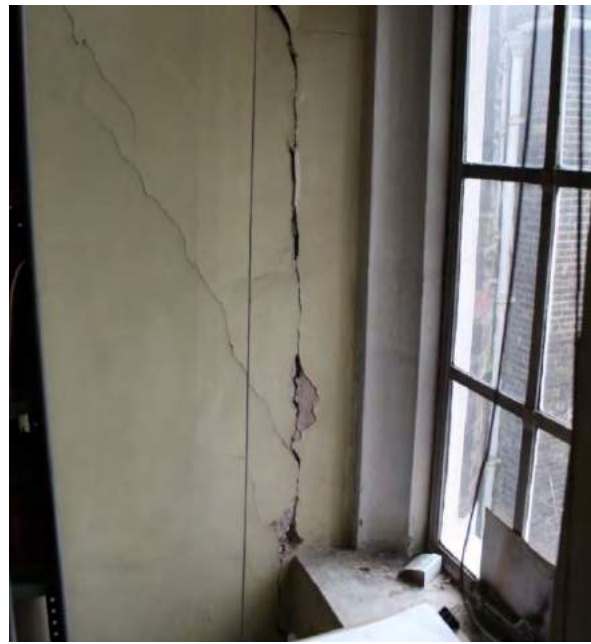
Figure 4: Cracking at internal partition walls (assumed loadbearing) where large floor deflections were observed
