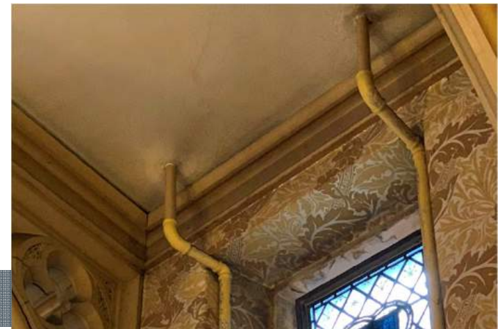
CONDITION SURVEY: Pipes running within stained glass window recess within Lecture Hall.
