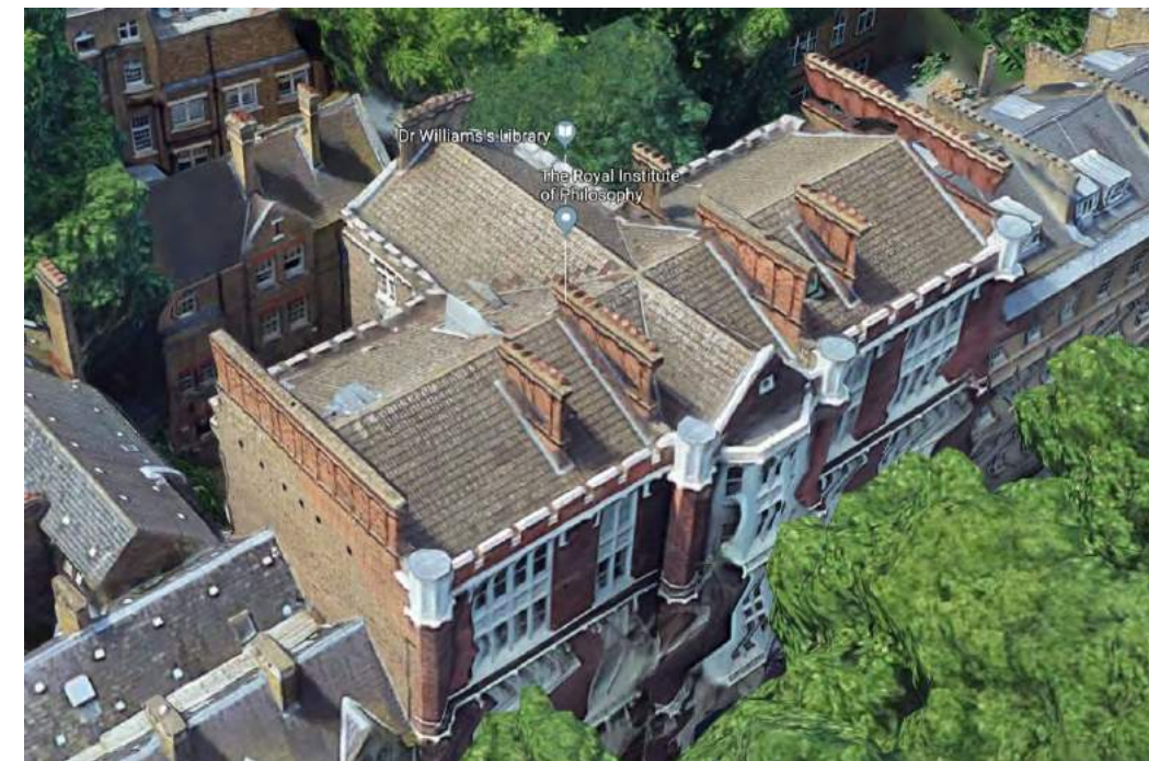
Figure 12: Roof of building from Google Maps. Steel discs visible at south wall
