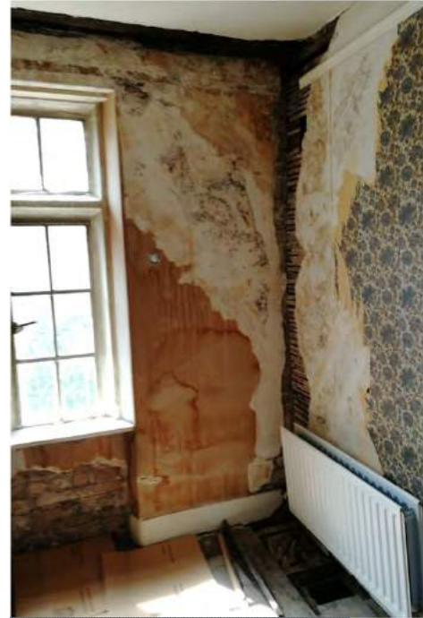
CONDITION SURVEY: Plaster damage and structural failings on level 7
