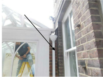
Vertical upward tapering crack at junction of the conservatory
