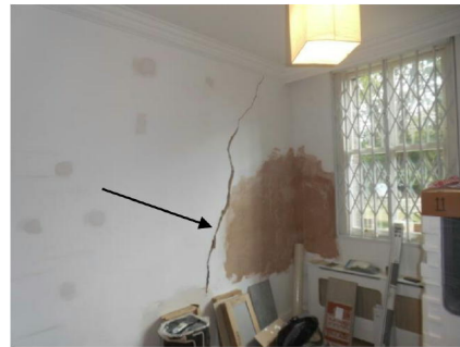
Structural crack to left partition in the rear middle room
