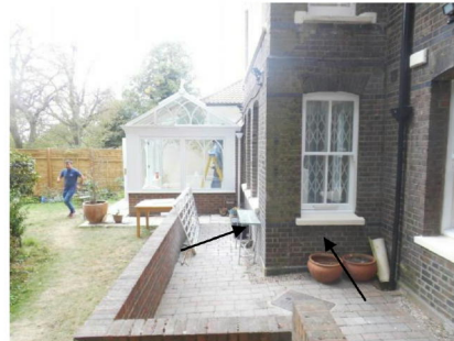
Bay structure and conservatory seen from the left – damage to brickwork at low level
