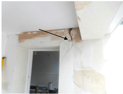
Cracks around door – conservatory/kitchen area leading to the rear right lounge
