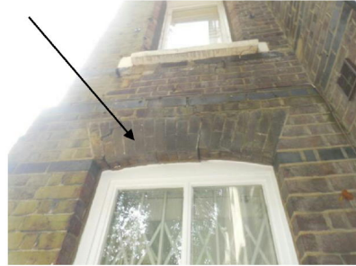
Damage to brick arch
