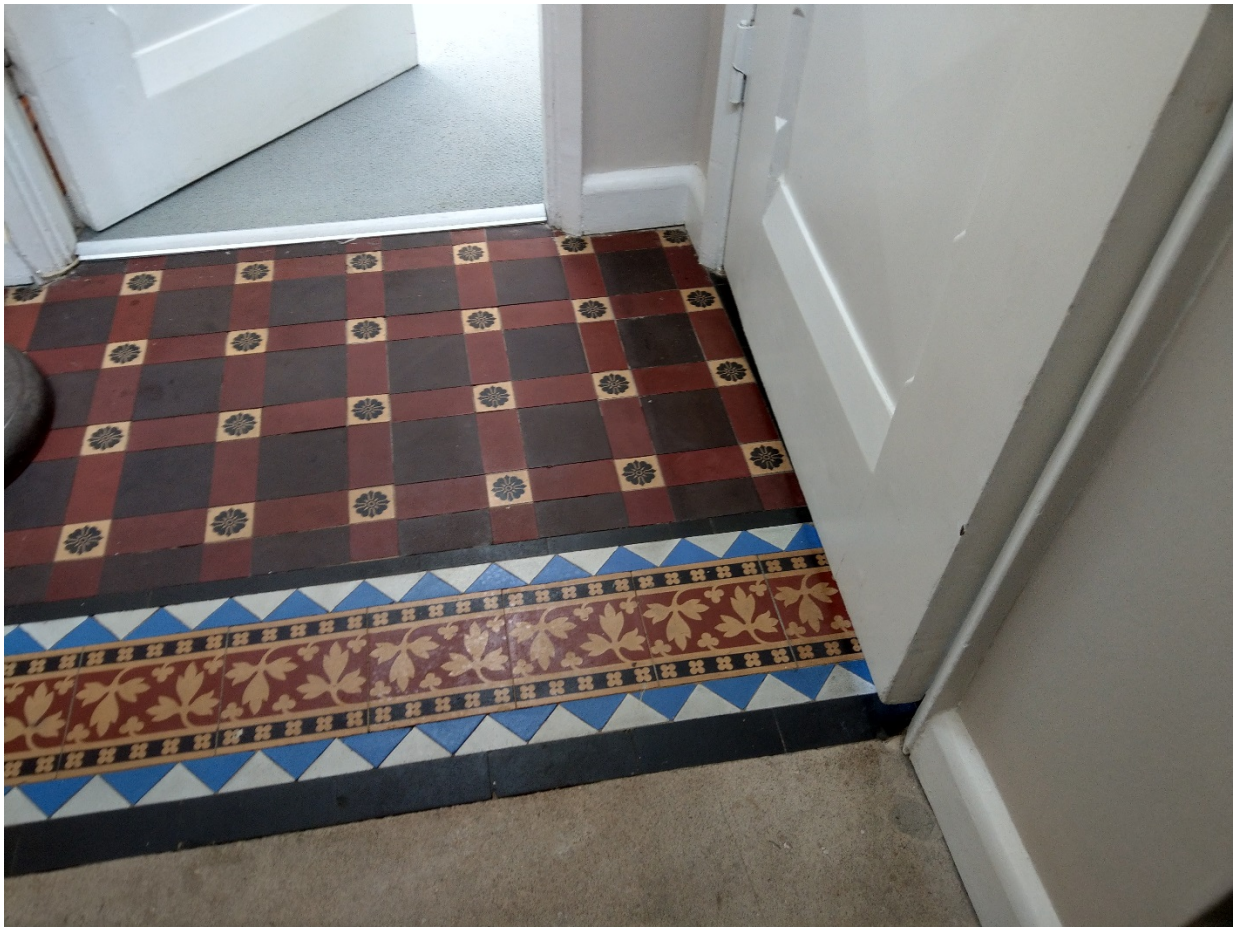
Figure 26 – Mezzanine landing - original Minton tiles retained, albeit opening up works show that these were unfortunately cut at the line of the bathroom and bedroom partitions, when they were created in the 1950s.
