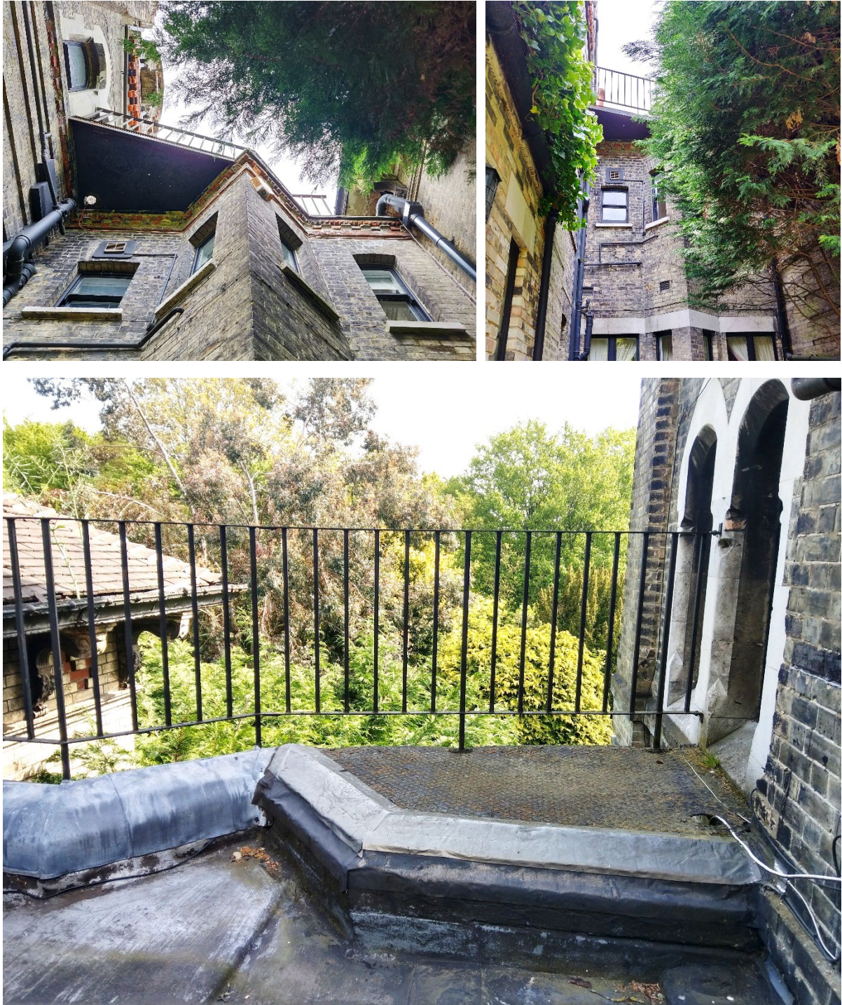
Figure 20 - View of existing roof terrace access - a metal landing bridges across from a tower window onto the roof terrace, with railings fixed into the top of the parapet. Proposal – remove unsympathetic bridge and metal balustrading. Provide alternative roof and maintenance access from the rear of the tower, where it will be concealed from view. Replace balustrading with a more sympathetic design that will not detract from the front elevation, set at the lower level of the roof terrace.
