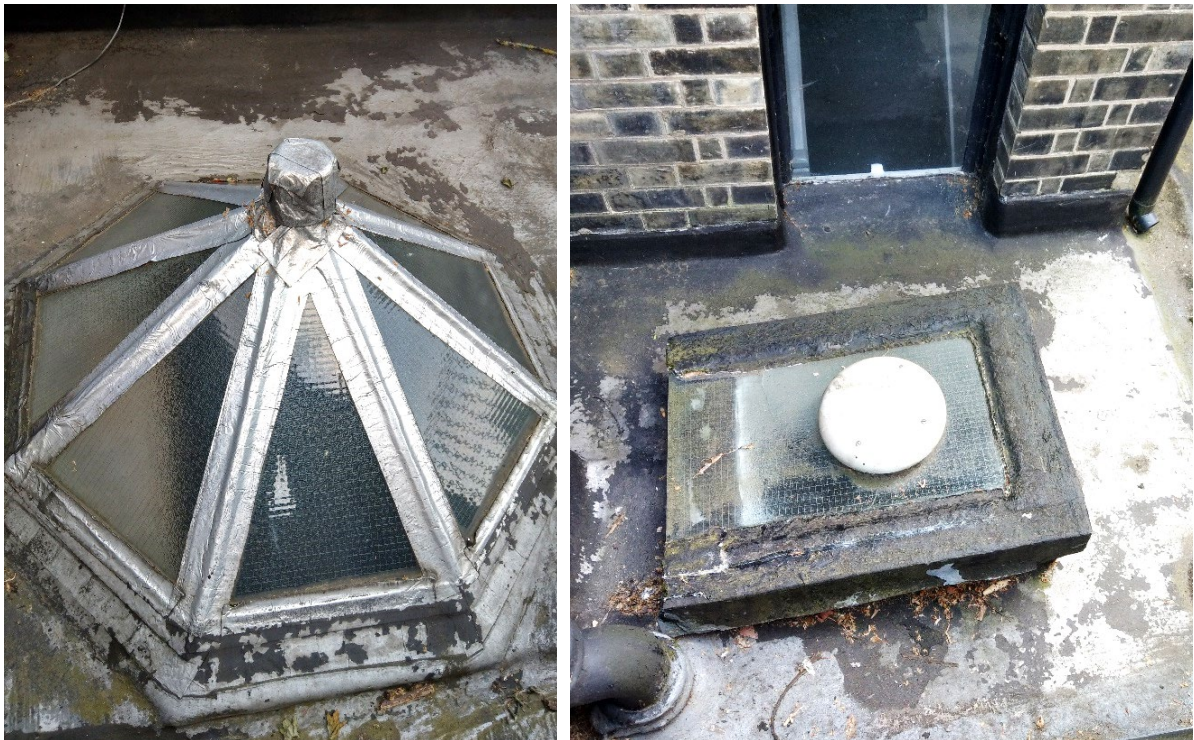
Figure 19 - Modern glazing and flashing to rooflights. LHS image - Proposals - remove modern glazing and Flashband and replace with clear, toughened glass to meet Part K requirements for protection from fall. RHS image - Proposals – rooflight to be removed and roof to be repaired accordingly.
