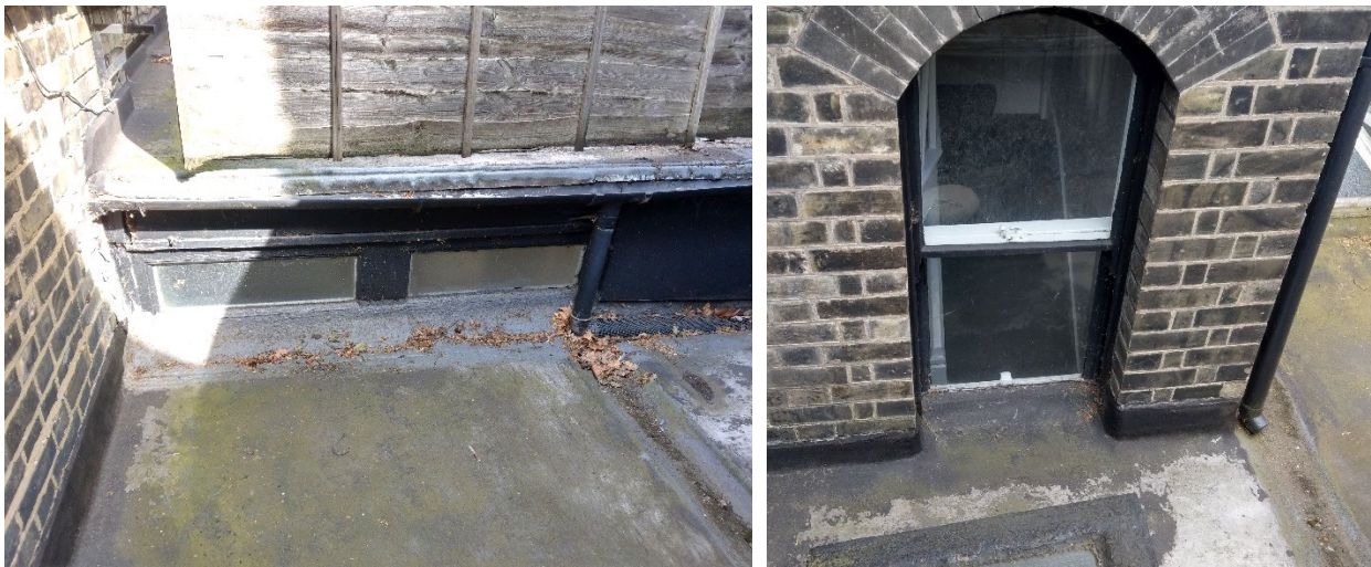
Figure 22 - Poor roof to glass detailing. Proposals - review roof waterproofing upstands and replace modern glazing with clear Part K compliant glazing to protect against fall. Window in RHS image – Proposals to raise opening to provide new access to roof and improve waterproofing junction.
