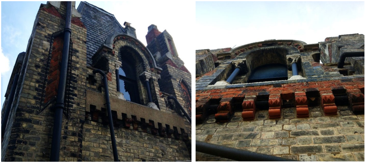
Figure 21 – LHS image shows unsympathetic cementitious render to rear elevation tower detailing. RHS shows original detailing to side elevation. Proposals – Brickwork to be repaired by specialist masonry conservator to match original detailing like for like.
