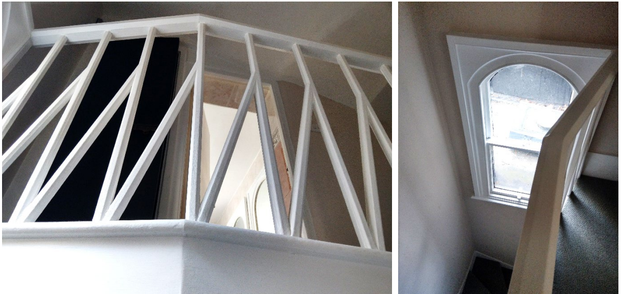
Figure 30 - Landing - 1876 Balustrade. Awkward junction between landing window (original) and 1876 extension roof. Poor waterproofing detail, with roof line hitting the glass above the window frame and cill. Window is concealed from all view except the roof terrace. This is the proposed location for the new roof maintenance access. Proposals – raise window opening and modify landing to provide door. Raising the opening will also improve the waterproofing detail on the roof side, with sufficient upstand to protect the brickwork and window from moisture damage.
