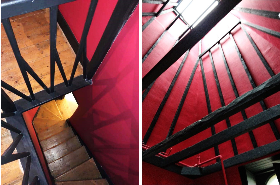
Figure 31 - Attic room and stair - Original staircase and timbers. Evidence of a previous mezzanine within the space (and ladder access notches). Modern rooflight at top of tower.
