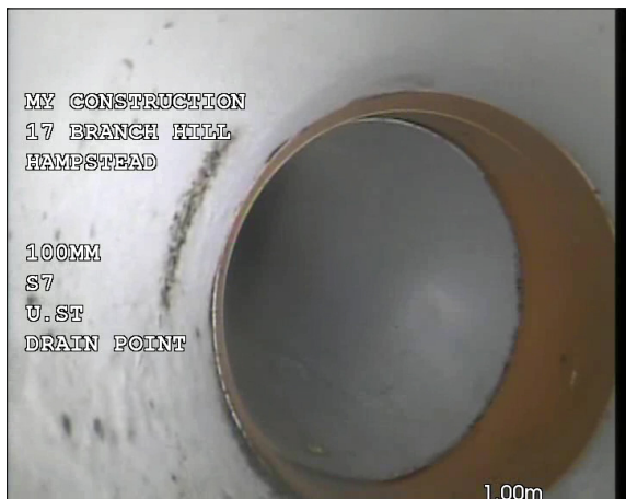
Photo: 13_6A, 00:00:01 1.22m, Line of sewer deviates left
