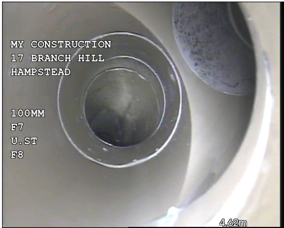
Photo: 4_6A, 00:00:01 4.62m, Junction, at 3 o'clock, 100mm diameter
