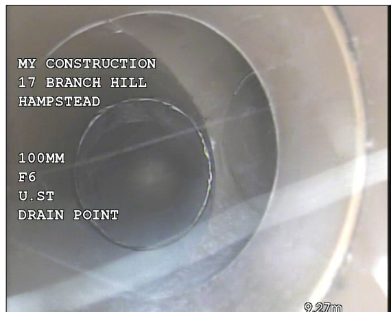
Photo: 1_4A, 00:00:01 9.22m, Junction, at 3 o'clock, 100mm diameter
