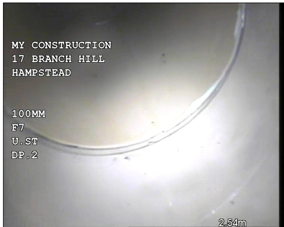
Photo: 6_5A, 00:00:01 2.54m, Line of sewer deviates up
