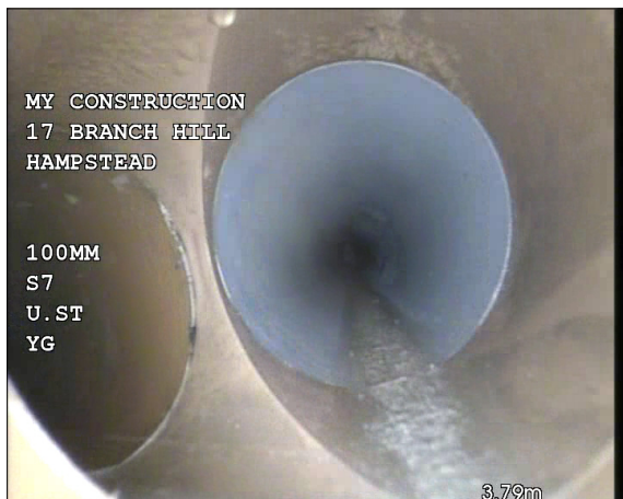
Photo: 14_5A, 00:00:01 3.79m, Junction, at 9 o'clock, 100mm diameter
