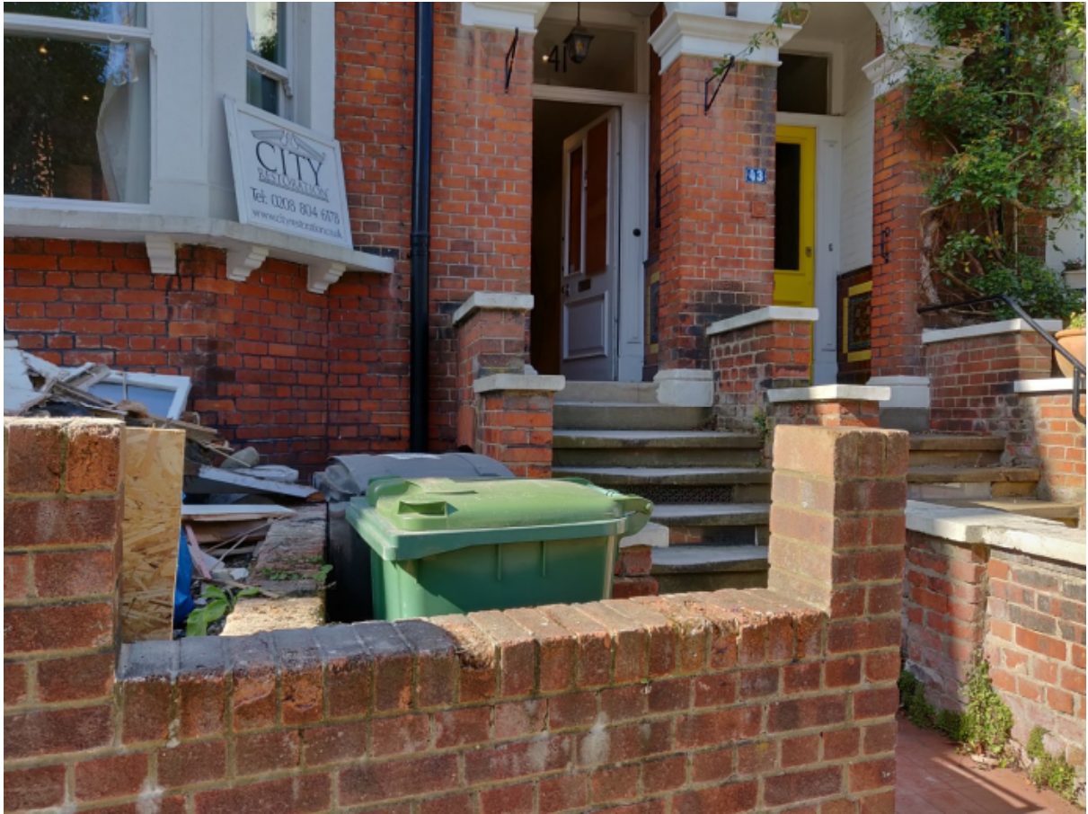
Photo 5: Front boundary wall to be rebuilt
