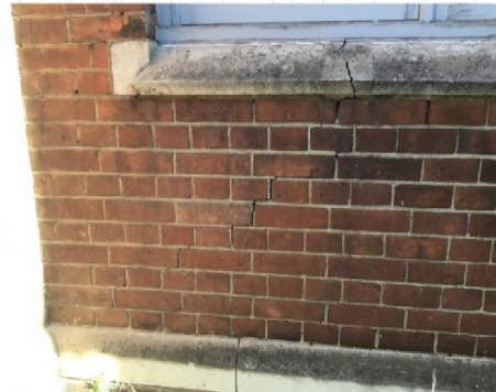
Crack To Left Flank Below Front Window
