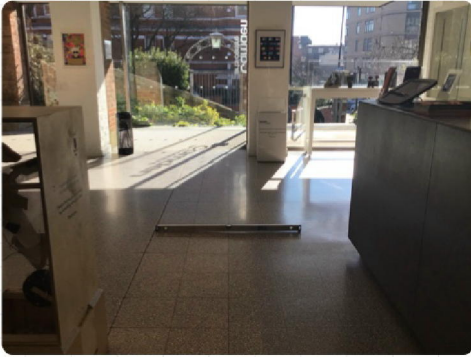
General View Of Movement Of Ground Floor In Front Entrance
