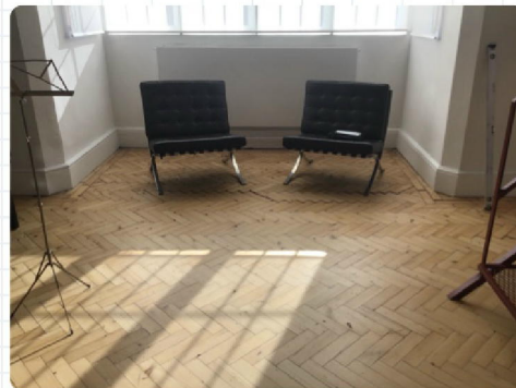
General View Of Crack To Floor To Front Section Of Gallery 3
