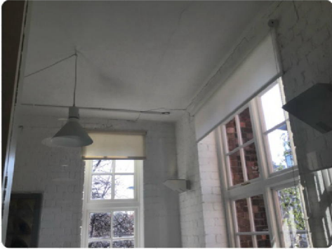
Cracking To Front Section Of Ground Floor Office
