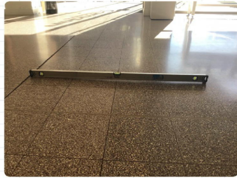
Close Up Of Movement Of Floor Of Ground Floor Front Entrance (Dropped 9mm Over 1200mm Length)
