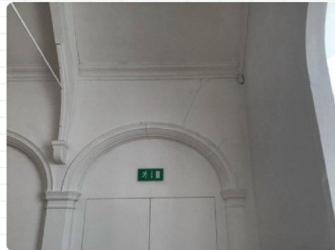
Crack Above Left Flank Internal Door In Gallery 3
