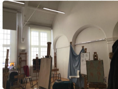
Crack Above Right Hand Door To Flank Wall Of Drawing Room
