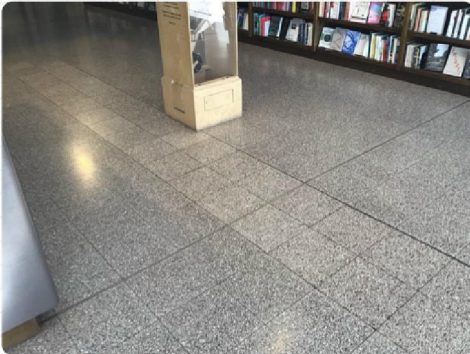
Previous Repair To Ground Front Entrance Floor In Same Area As Current Movement
