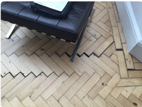
Close Up Of Cracking To Floor To Front Of Gallery 3
