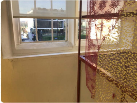
Crack Below RH Flank Window In Gallery 3
