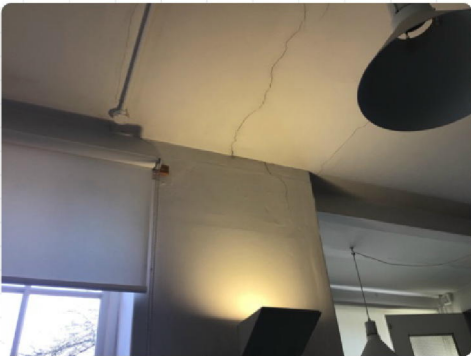
Cracking To Left Flank In Rear Main Ground Floor Office
