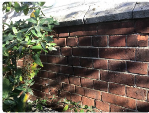
Crack To Left Flank Below First Bay Window
