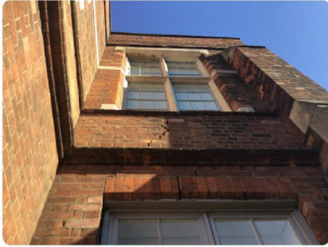
Crack To Left Flank Above Front Window
