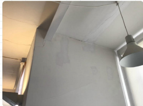
Cracking To LH Flank In Ground Floor Office
