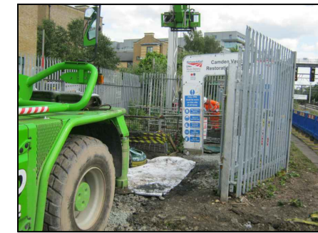
PHOTO 2 - VIEW OF ACCESS FENCING CURRENTLY SURROUNDING COLLAPSED ROOF
