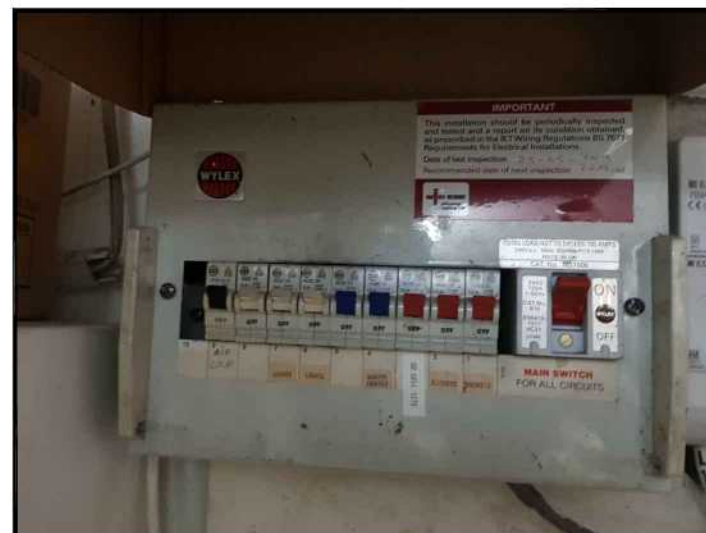
EXISTING LANDLORD DISTRIBUTION BOARD
