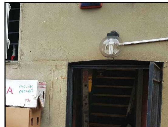
EXISTING LIGHT FITTING NEAR THE PROPOSED EQUIPMENT
