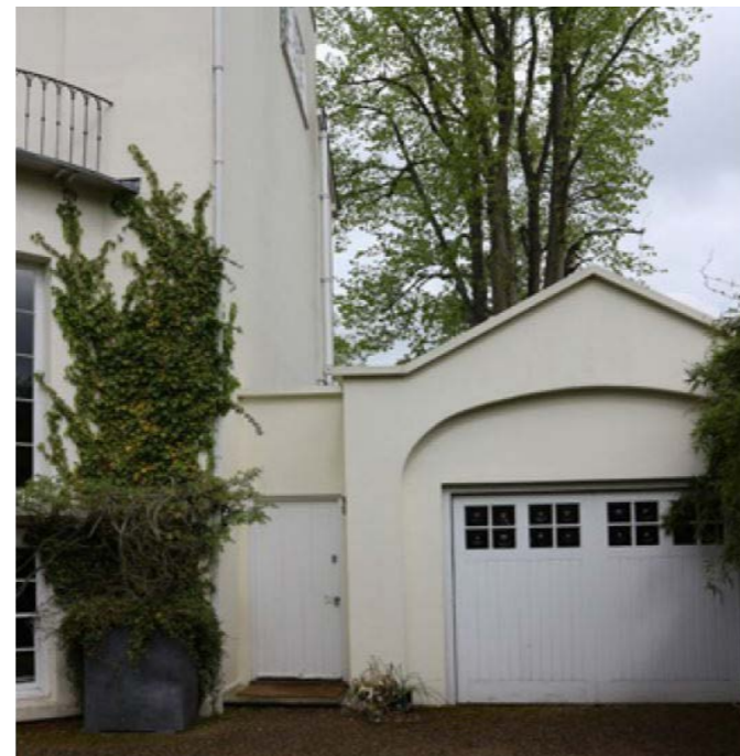
4. Garage Side Extension - poorly executed
