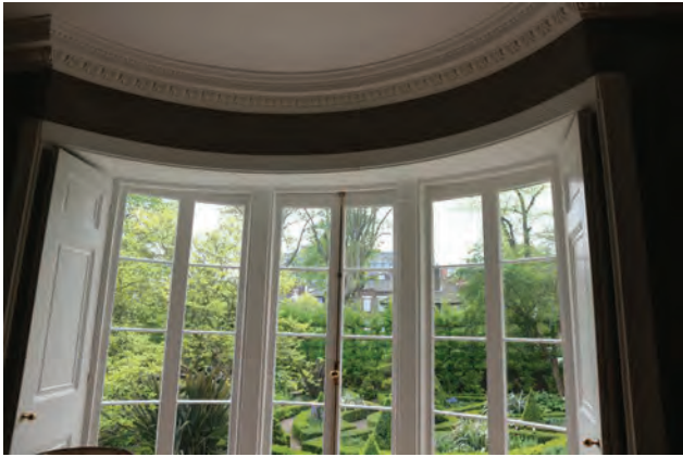
3.23 G5, leaning window opening in sitting room (Insall).
