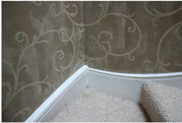
3.15B Mismatched string to principal stair at upper floors (Install)
