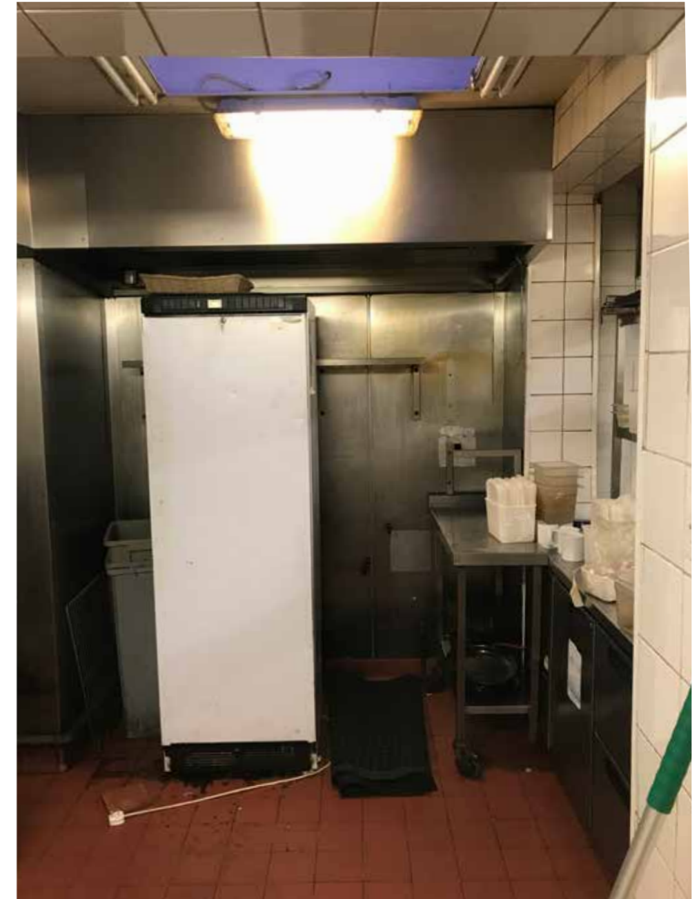
Existing kitchen at the rear of the ground floor, with roof light above
