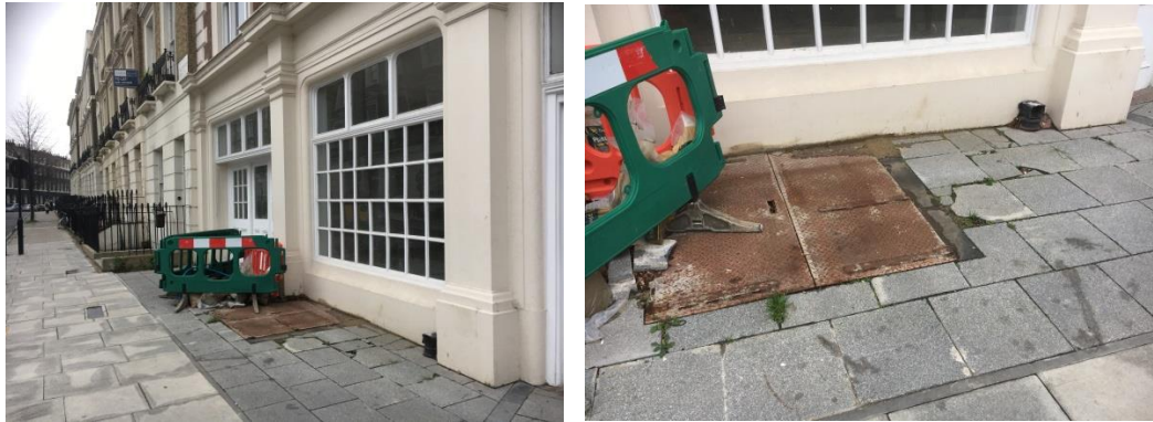
Figure 3.4: Functional / utilitarian barrel hatch set within the modern concrete paving around the former pub.
