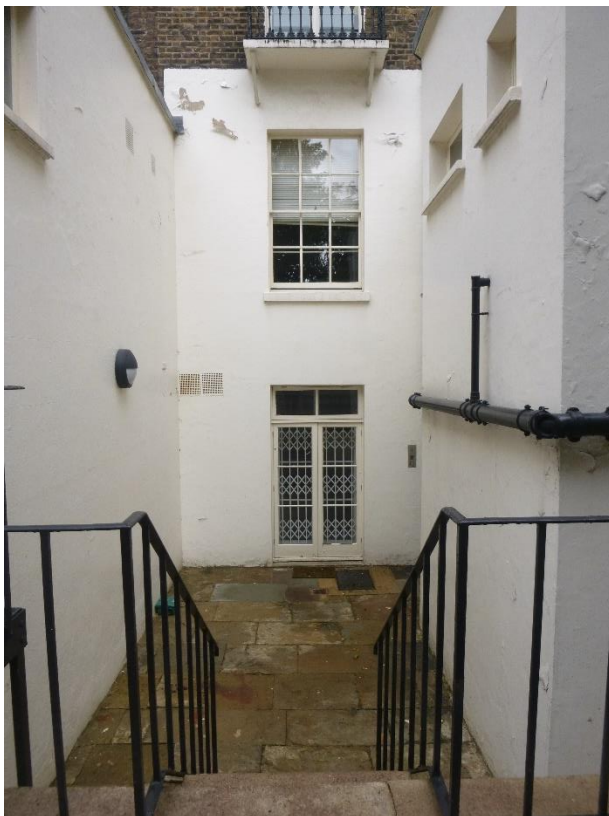
Fig. 12: Rear elevation of No. 56; a basement window opening has been converted into a doorway
