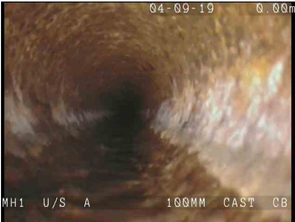
A_MH1X_7069cf84-8557-4d21-aaf6-a844871a4e0a_20190906_100331_033.jpg, 00:00:03, 0.10 m Attached deposits, encrustation from 12 o'clock to 12 o'clock, 5% cross-sectional area loss, start
