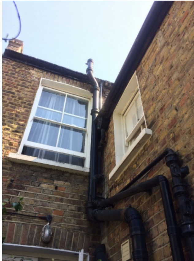
5. Existing window in side wall of rear return to now be retained.
