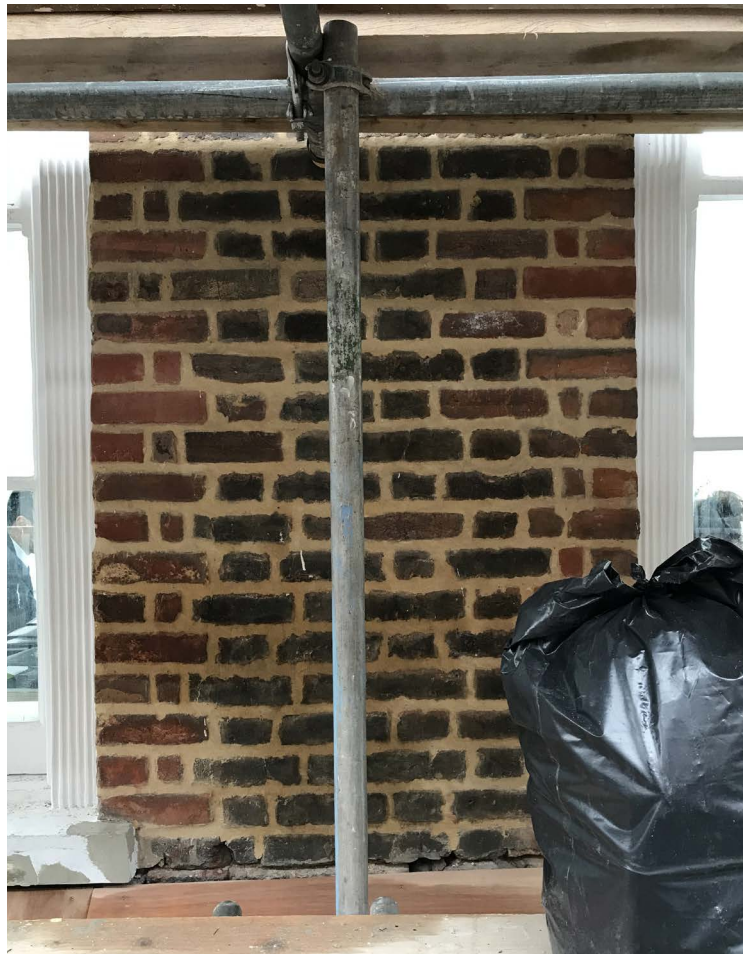
No. 5 Great James Street Unsympathetic cement re-pointing.
