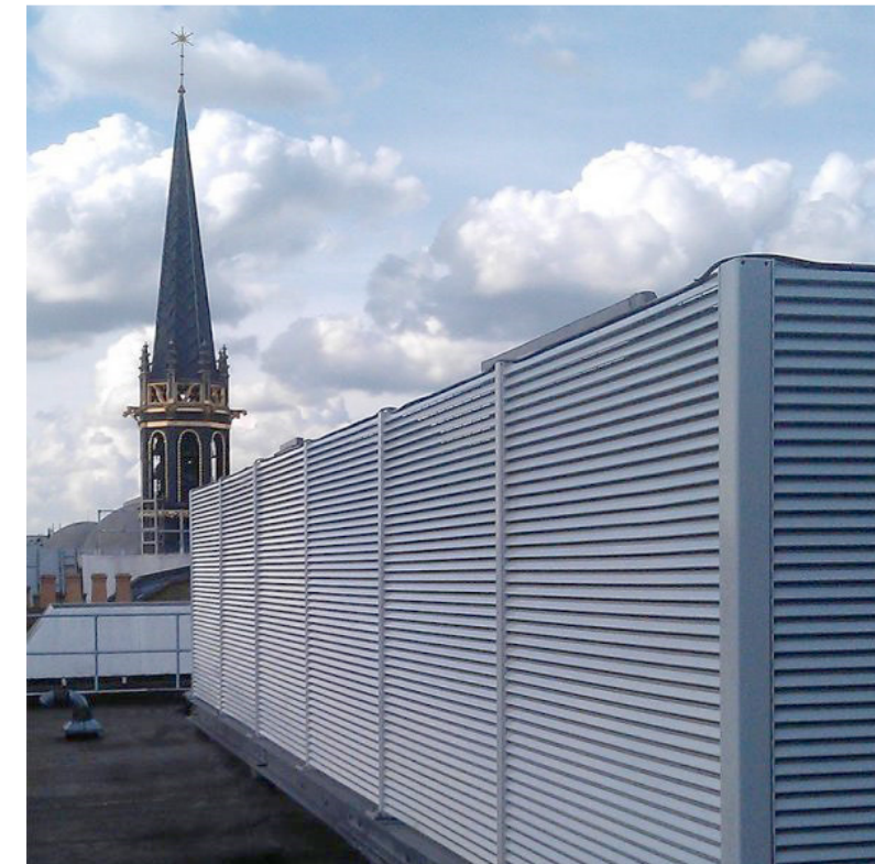
Louvres to Roof Mounted Plant Enclosure
