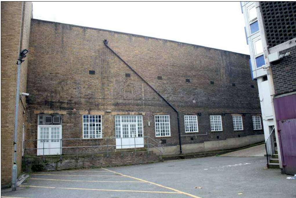
Plate 34: View of the north elevation of 'The Place' (Grade II listed) as visible from within the Site car park/service yard
