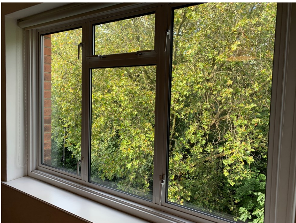
Close up of existing 3 panel window (note: no glazing bars in existing uPVC window)
