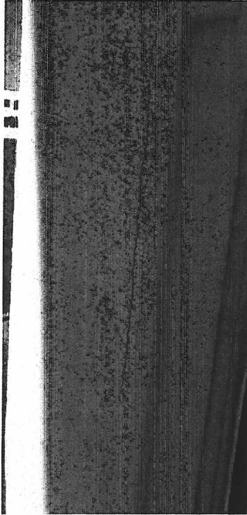
Pic 5 – Typical crack around window frames
