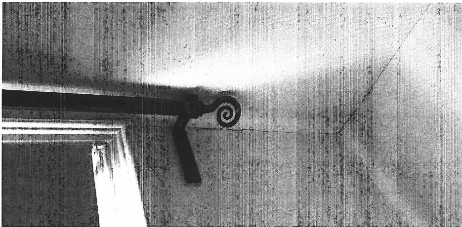
Pic 6 – Internal crack at ceilings
