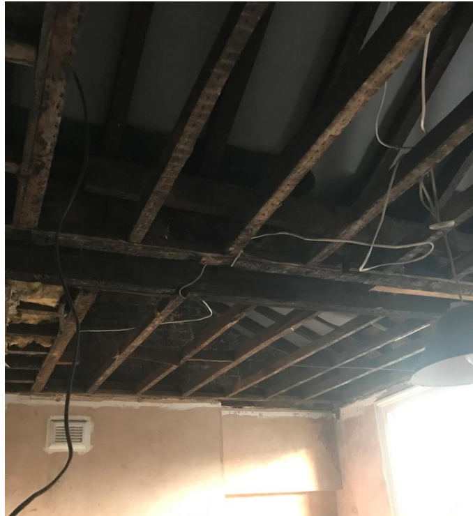
Fig. 8 Photo of rafters taken by client before they became inaccessible
