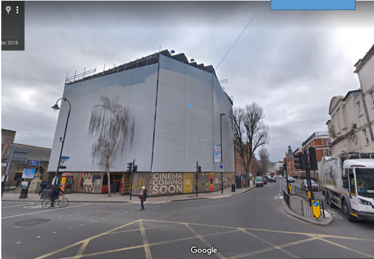
Photo 1 (above): View of the site with the scaffold and shroud already in place. The commercial advertisement is to go on the apex elevation.
