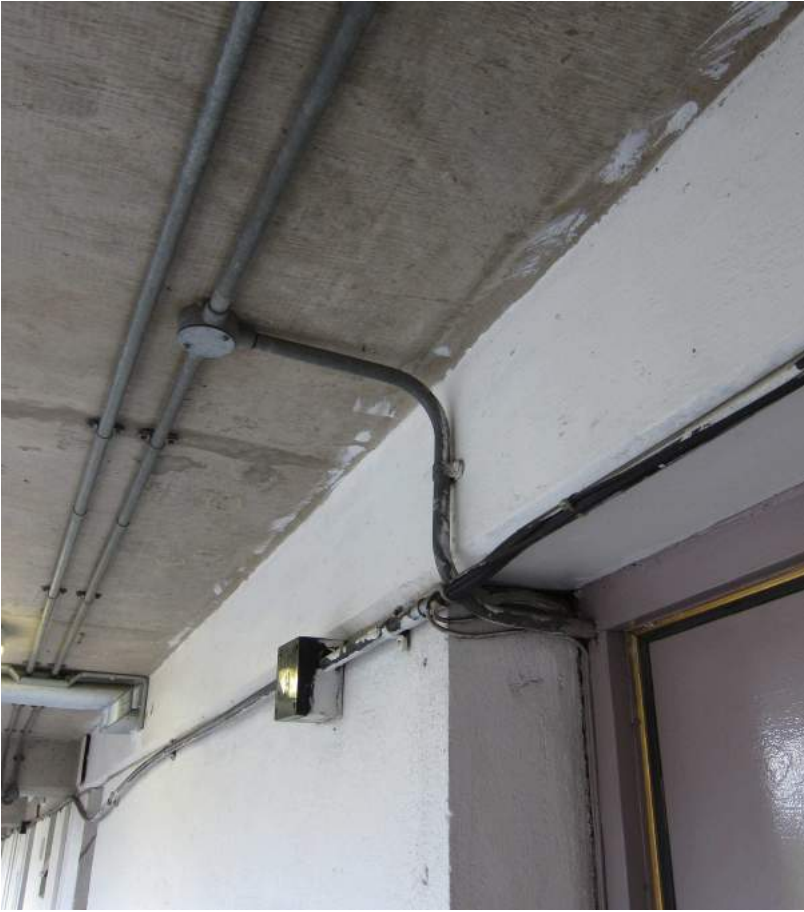
Existing door entry system round conduit, with entry through head of door frame
