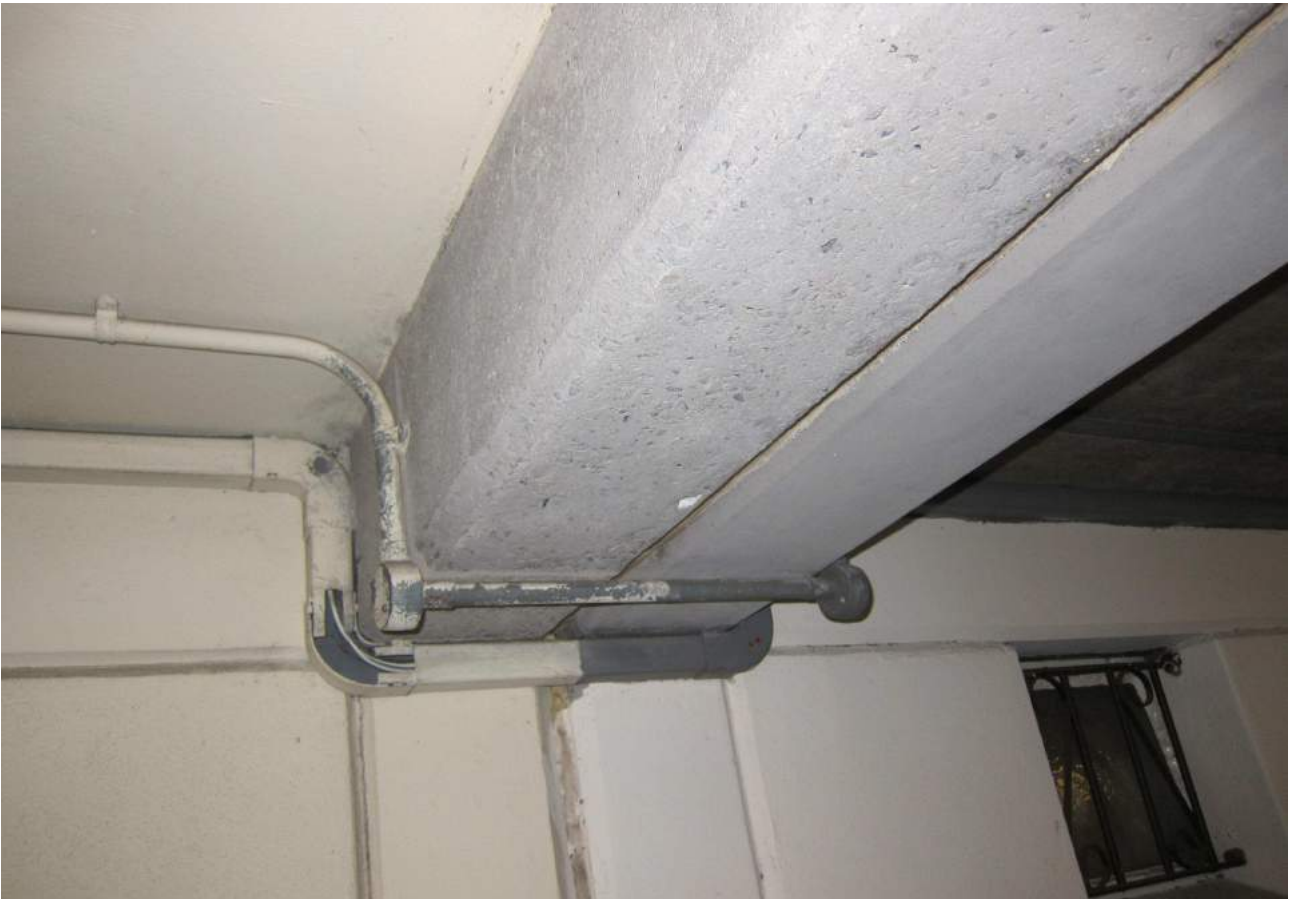
Round door entry system conduit, with square section conduit behind
