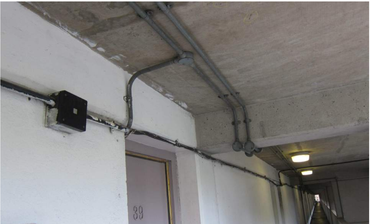
Existing door entry system round conduit, with entry through head of door frame
