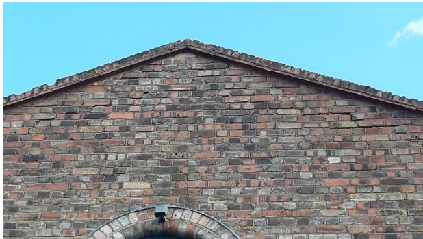
Plate 3.3 Cracks in Brickwork Near Roof
