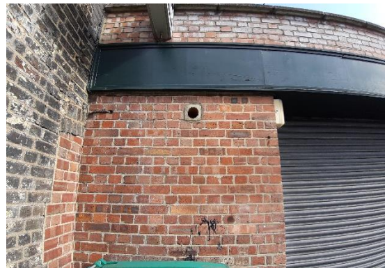
Plate 3.6 Gap in Brickwork for Pipe
