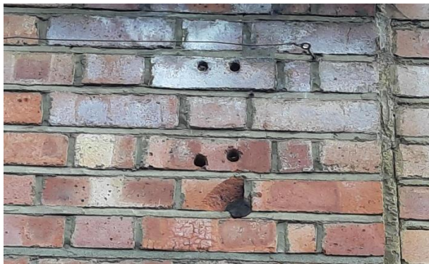
Plate 3.5 Holes in Brickwork
