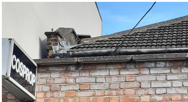
Plate 3.7 Lifted Lead Flashing
