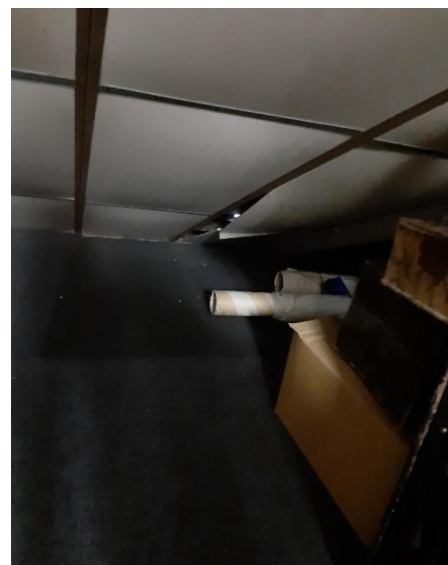
Plate 3.17 Damaged Roof Panels
