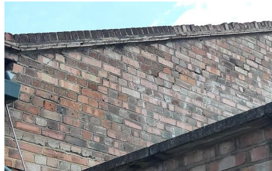
Plate 3.4 Cracks in Brickwork Near Roof
