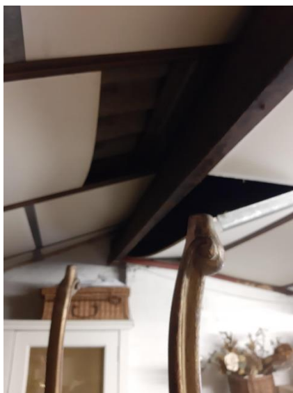
Plate 3.16 Lifted Roof Panels
