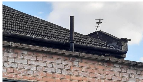
Plate 3.8 Lifted Lead Flashing
