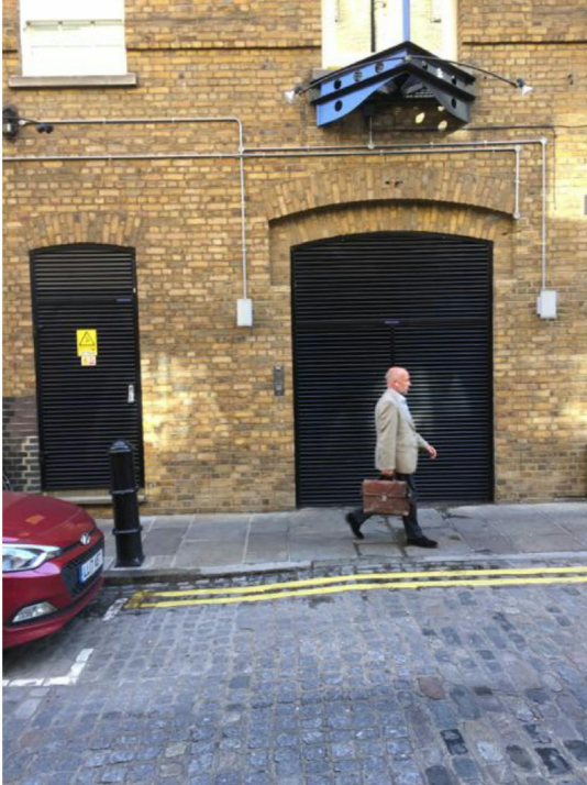
Photo 4 This photograph of part of the Thomas Neal development in Shorts Gardens. The louvred door to the right serves the electricity substation and gives 24 hr emergency access and fresh air ventilation to the substation. The substation is noiseless and the extent of the louvre is plainly just a door width and there is no extraction/intake of air. The double louvred doors to the right give access to the store room of the street cleaning machines see photo 5 below.
