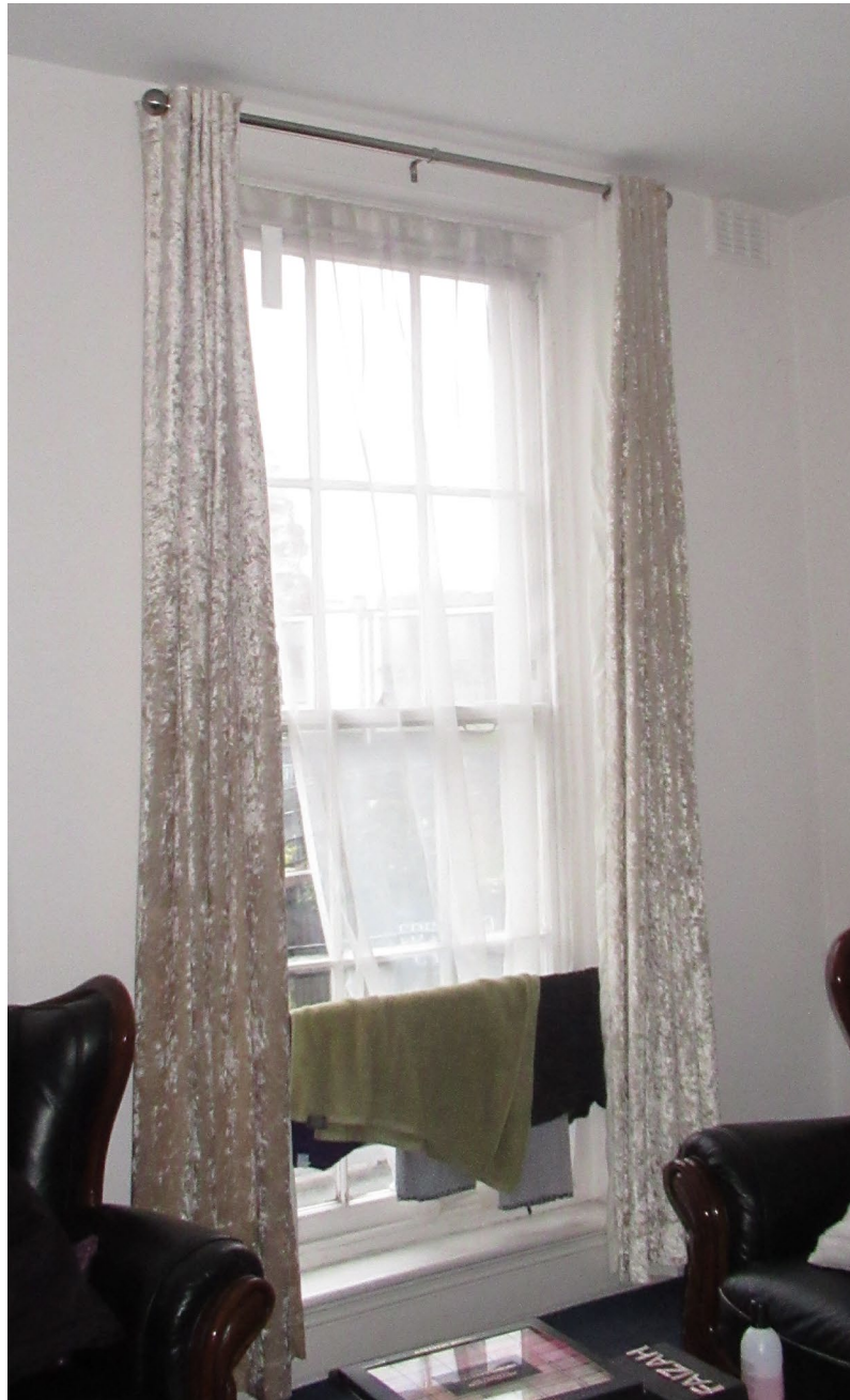
Figure 10: Internal view of right hand side window at first floor level – living room
