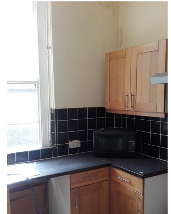
Fig. 17 1st Floor Kitchen units to be replaced
