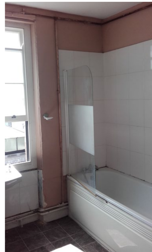
Fig 20. Existing bathroom to be upgraded and rear window to be replaced to match existing
