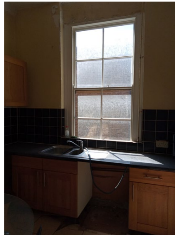
Fig. 16 1st Floor rear window to kitchen to be replaced in existing opening
