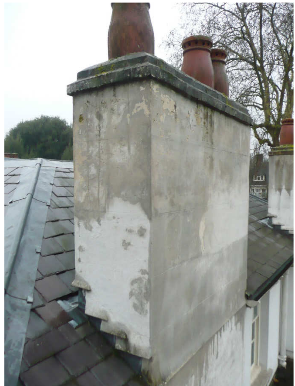
Fig. 16: South East Chimney during rain
