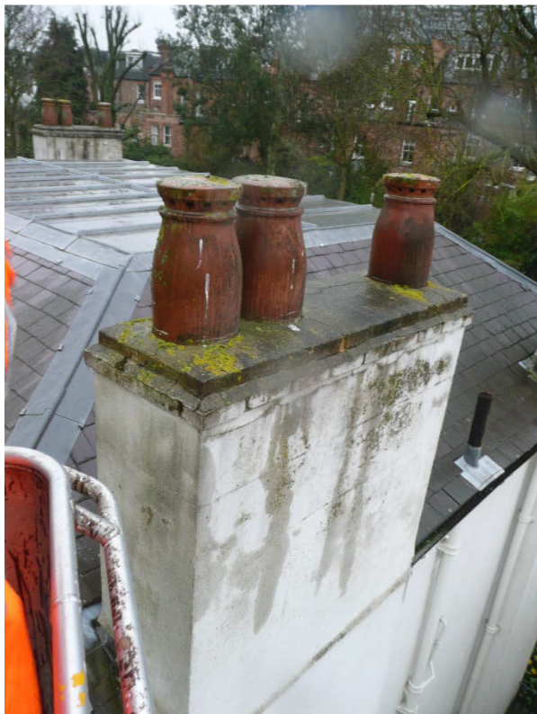
Fig. 15: North West Chimney during rain
