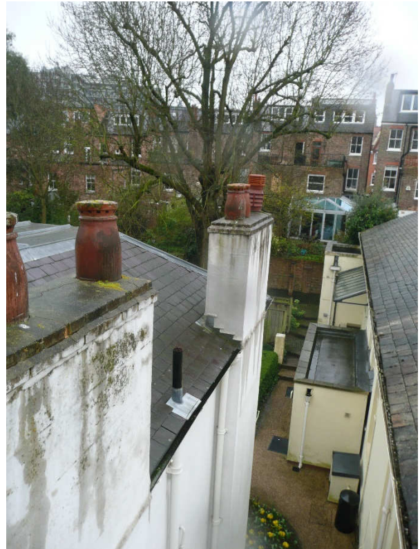
Fig. 14: West Elevation of Western Chimneys during rain
