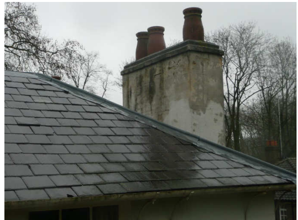
Fig. 12: West Elevation of South West Chimneys during rain
