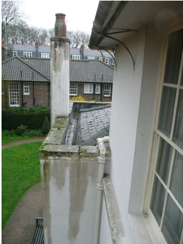
Fig. 13: Annex Chimney during rain
