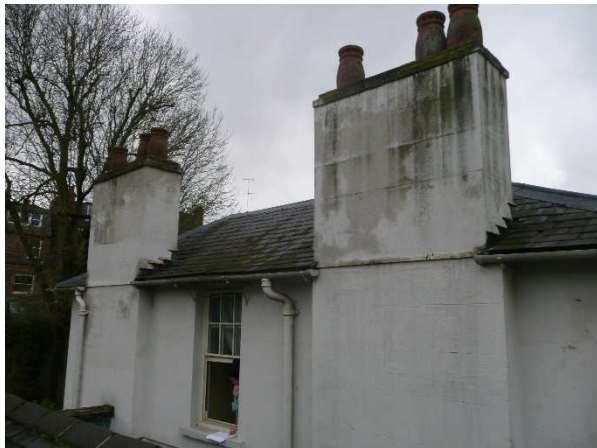
Fig. 11: East Elevation of Eastern Chimneys during rain
