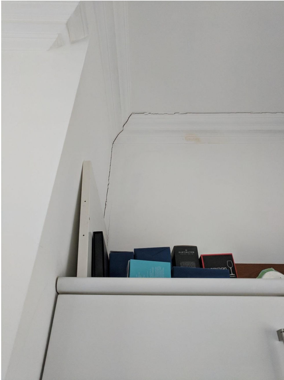
Photograph 4 - Internal crack at ground floor level
