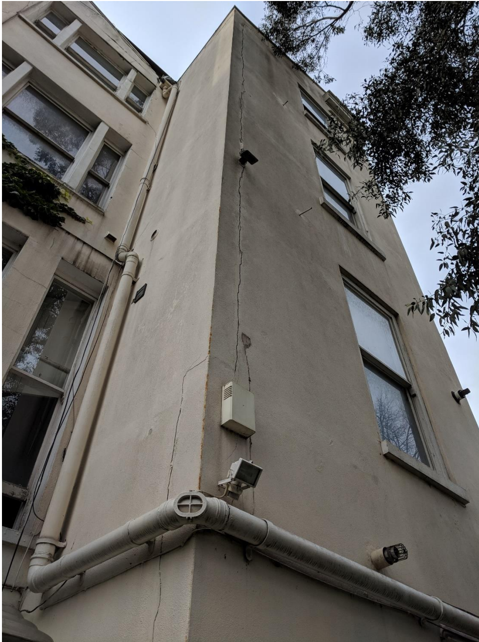
Photograph 5 - External crack to rear extension
