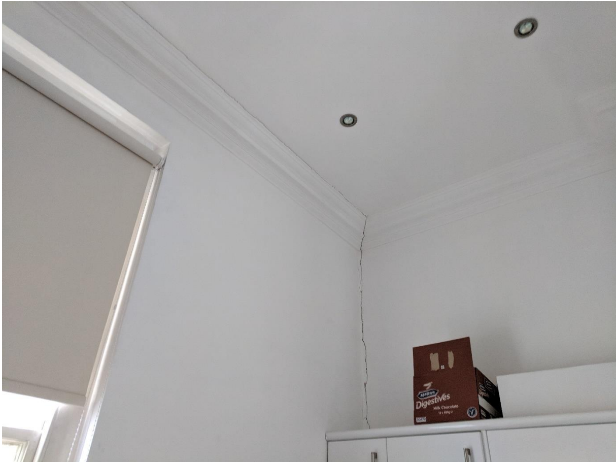
Photograph 6 - Internal crack at ground floor level on junction of rear and side wall
