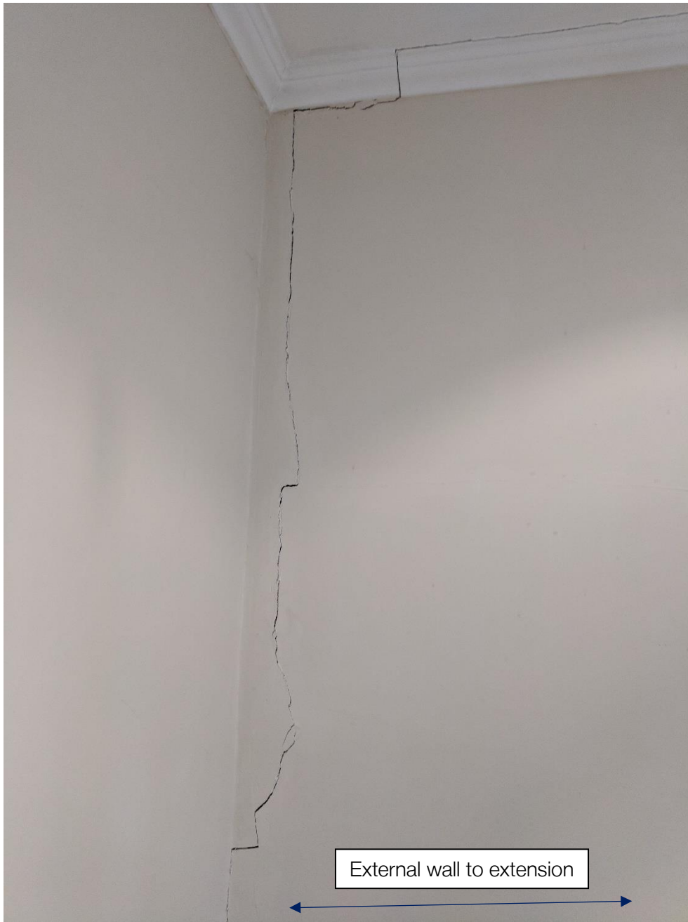
Photograph 3 - Internal crack at lower ground floor level
