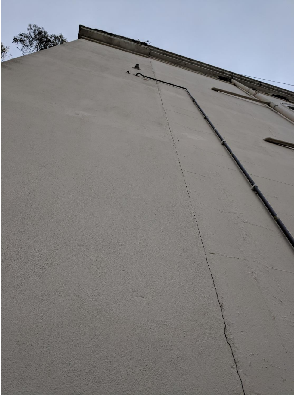
Photograph 2 - Cracking between original house and extension
