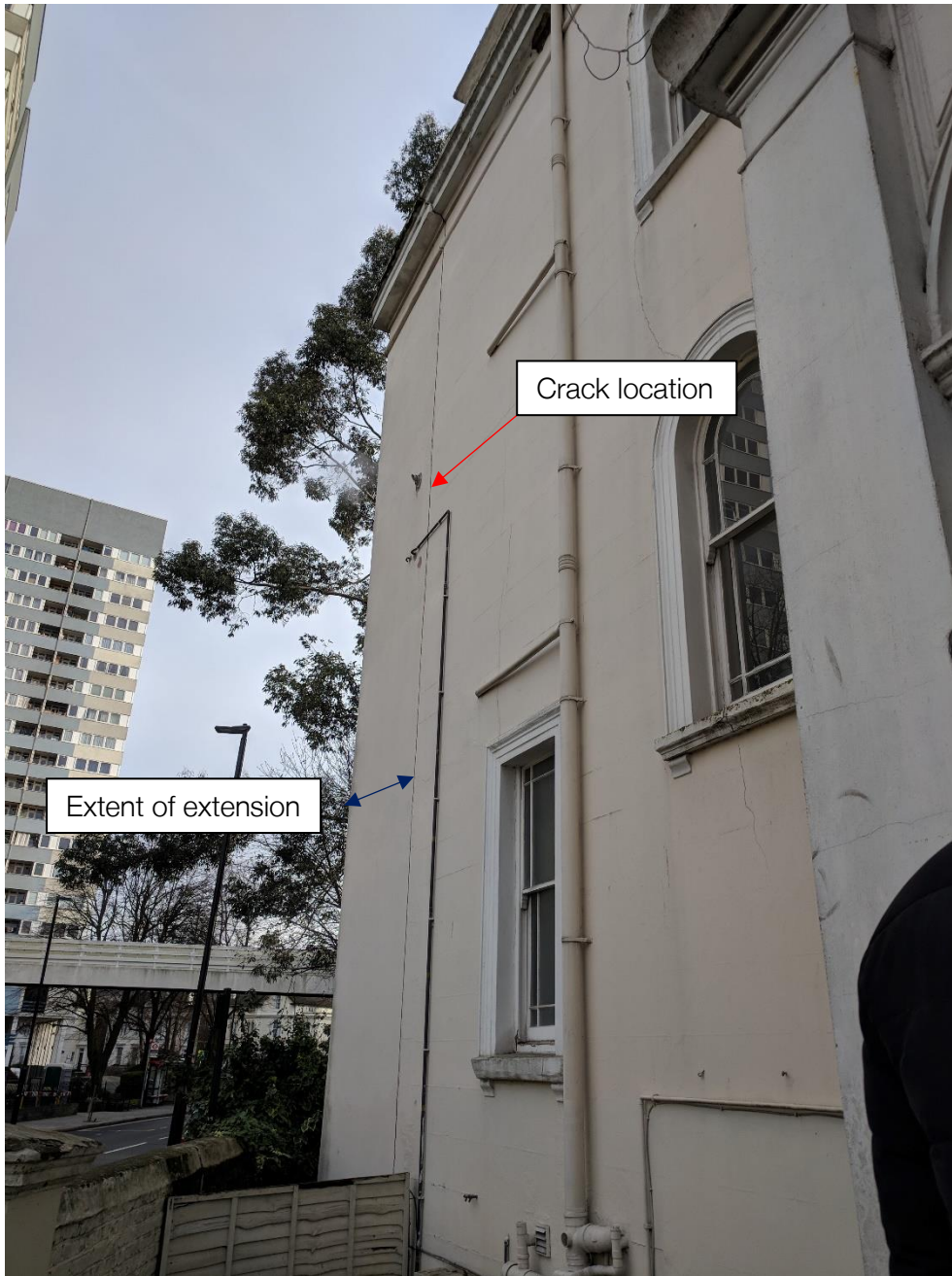
Photograph 1 - Cracking between original house and extension
