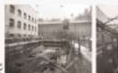
William Abney's sub-station (Brain Yard) under construction. The location of Panther House can be seen to the right.
