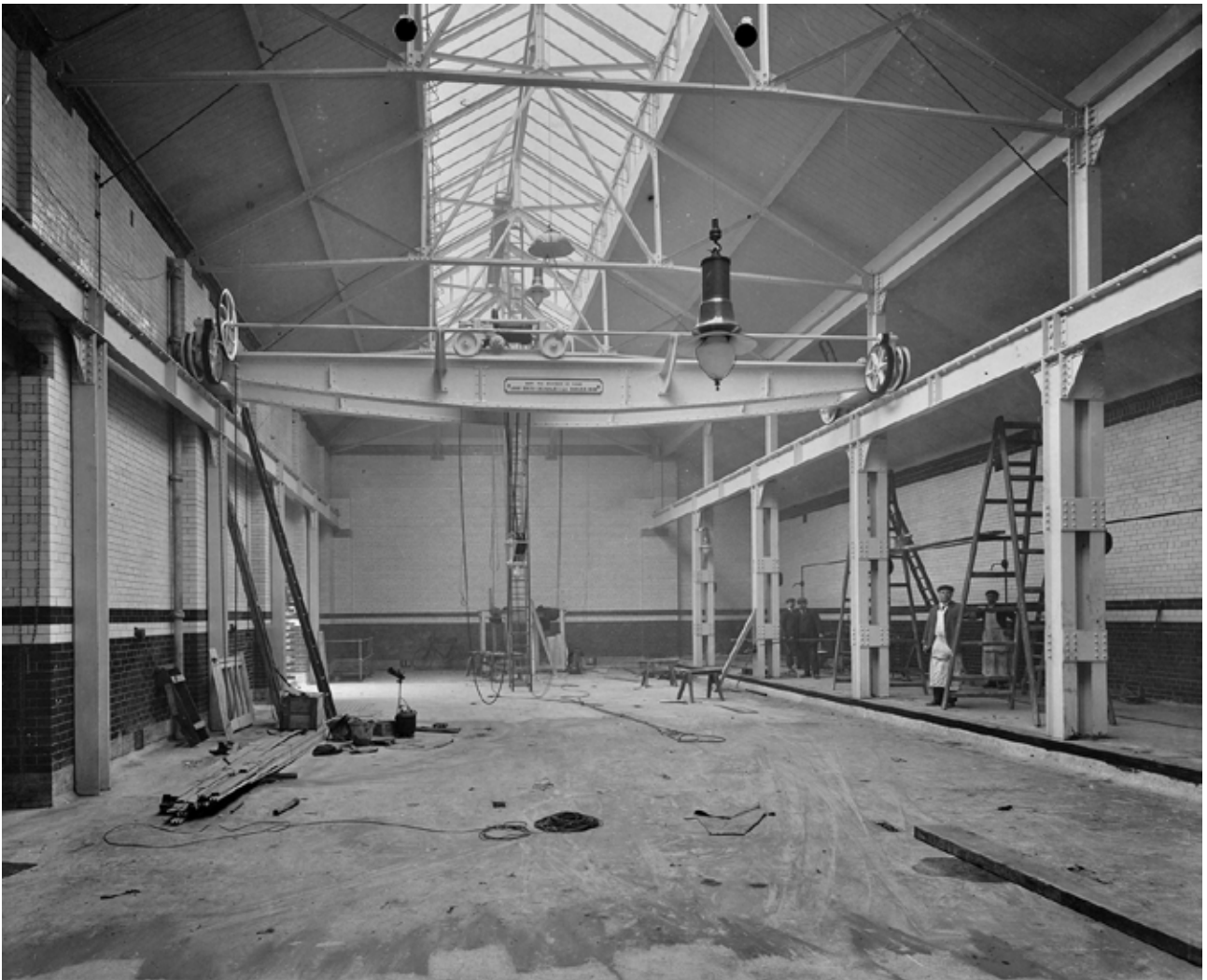
32. Interior of the nearly-completed Holborn substation, 1907 (Collage)
