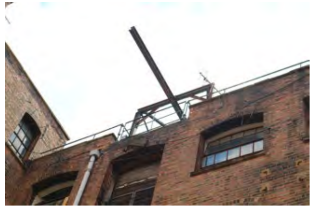
57. Detail of Block A showing the 1950s electric hoist on the roof level and shuttered opening below (Insall, 2018)
