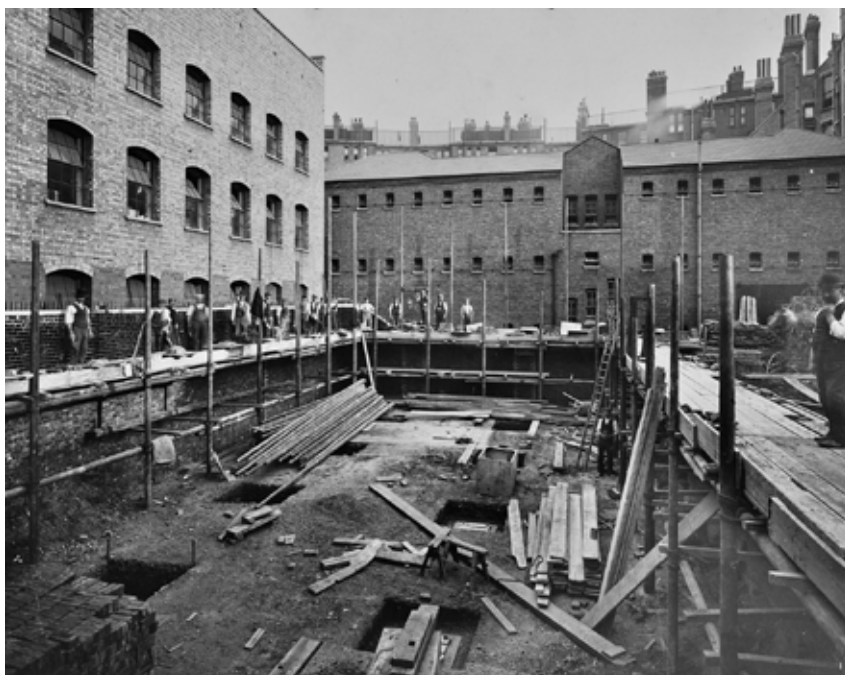
11. Holborn substation during construction showing the west wall of Malby & Sons new premises, 1906 (Collage)
