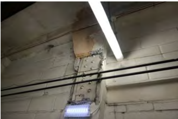
71. Submerged column in basement, Panther House (Insall, 2018)
