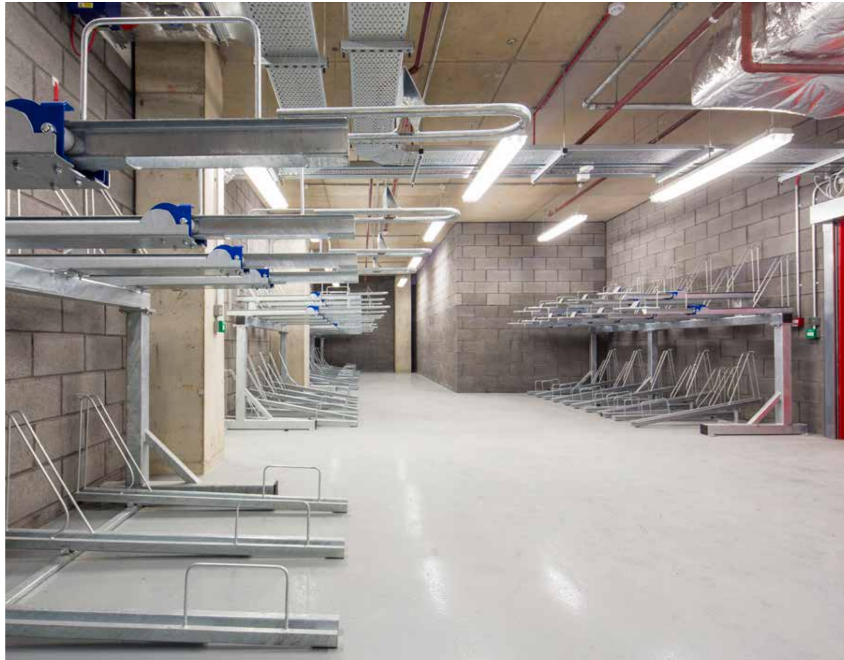
Figure 18: Photo of the cycle parking in the Building B4 basement on completion
