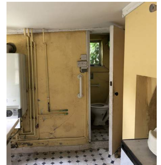
Interior of the existing extension at the rear of the property which is currently in poor condition.
