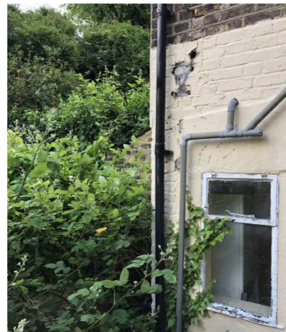
Current mixture of windows, painted and non painted brickwork and pipework on the existing building.
