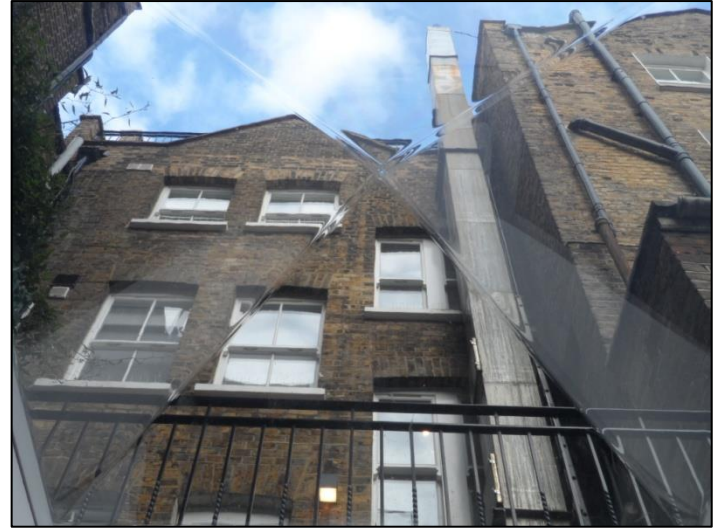
Figure 3 – Exhaust duct to be replaced.
