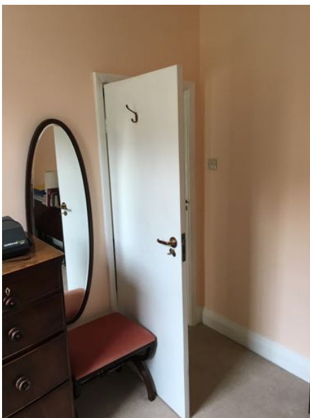
PHOTO 1. Back room showing First Floor dividing wall to RHS before mortar removed.
