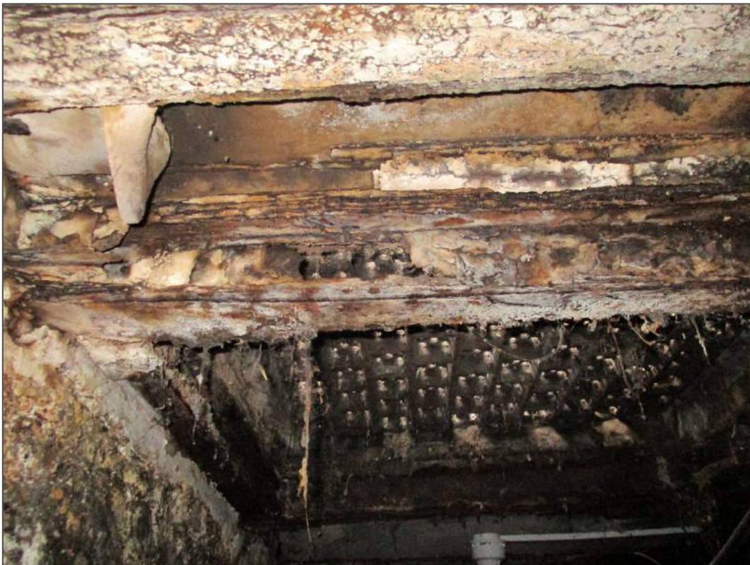
Photograph 14 – Corroded pavement light trimmer beam in basement south (2)
