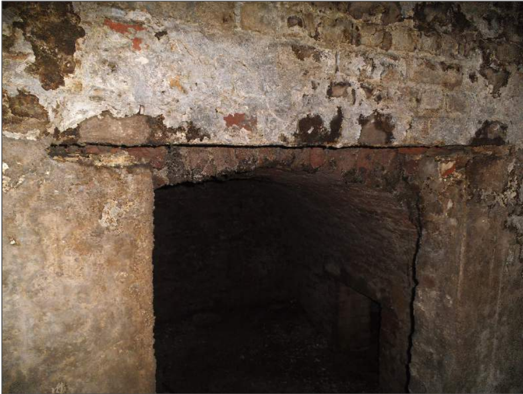
Photograph 27 – Missing lintel in basement west
