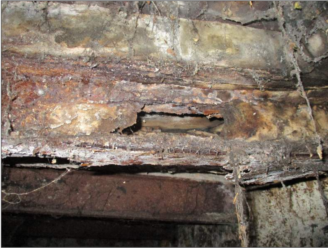
Photograph 13 – Corroded pavement light trimmer beam in basement south (1)
