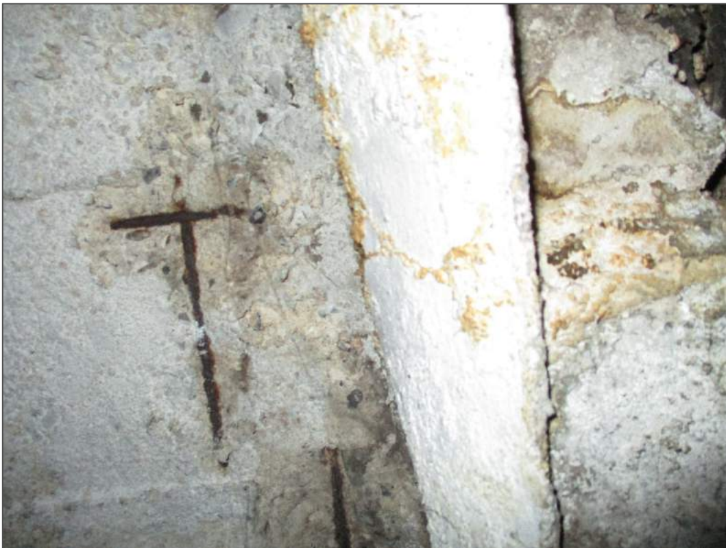
Photograph 16 – Exposed and corroded reinforcement in RC slab in basement south
