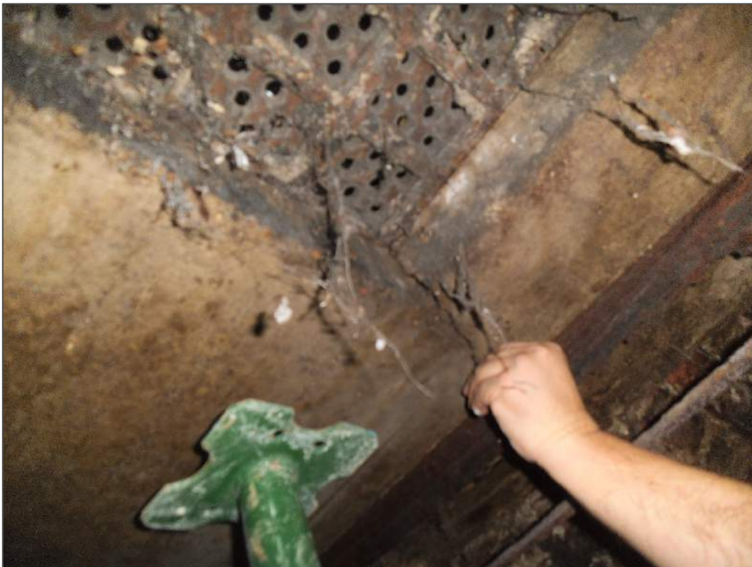
Photograph 24 – Crack in ground floor slab soffit, basement west
