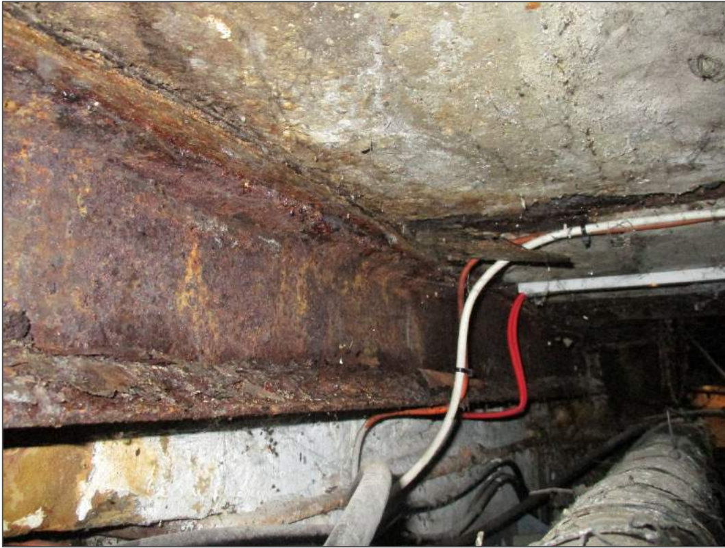
Photograph 11 – Corroded primary beam in basement south
