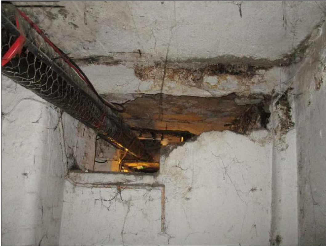
Photograph 17 – Opening in masonry wall in basement south
