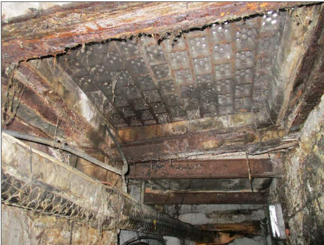
Photograph 12 – Corroded beams in basement south
