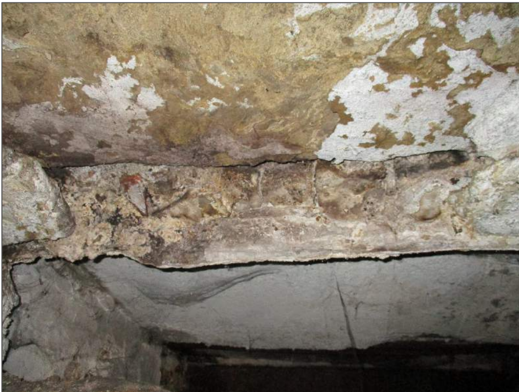
Photograph 18 – Unsupported brickwork over opening in basement south
