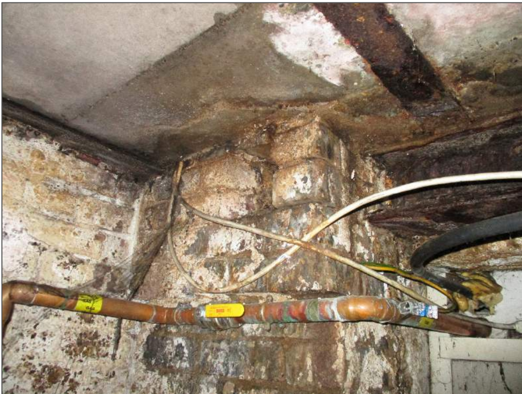
Photograph 10 – Masonry pier with missing bricks in basement south
