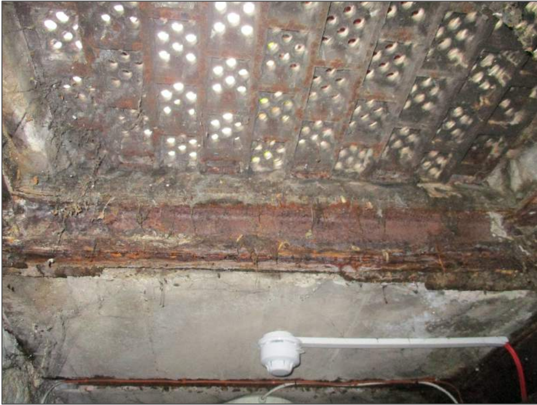
Photograph 15 – Corroded pavement light soffit
