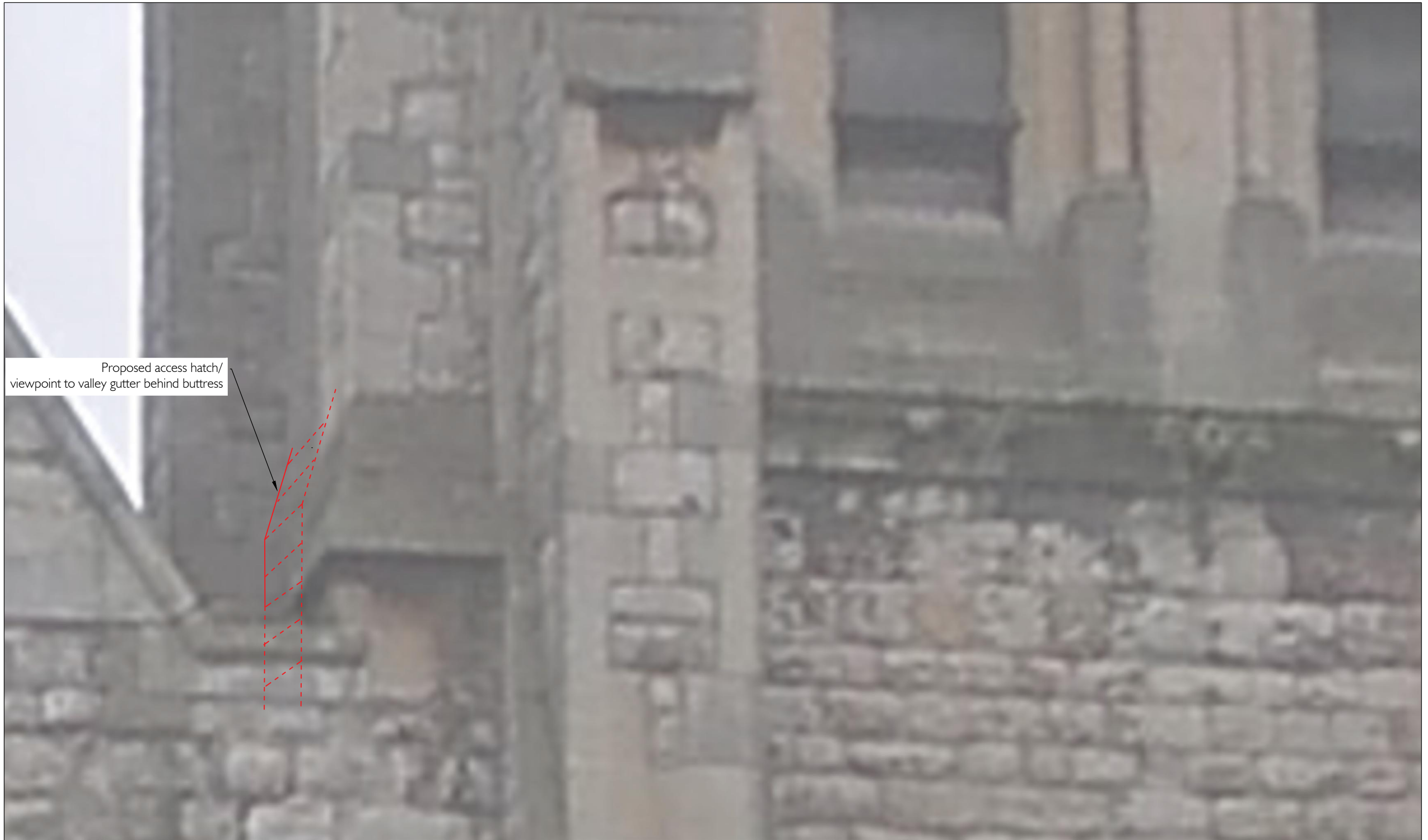
West elevation showing location of proposed access to valley gutter by inserting a hatch in place of the bottom louvre
