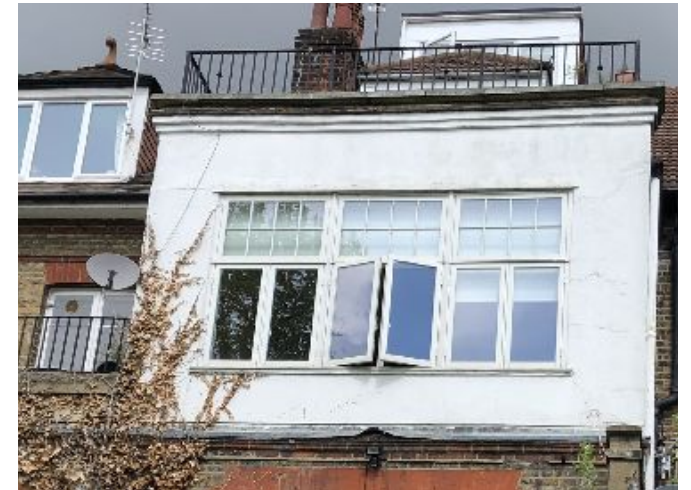
24. Existing render band to client's apartment and where opening up of window (below sill) is proposed.
