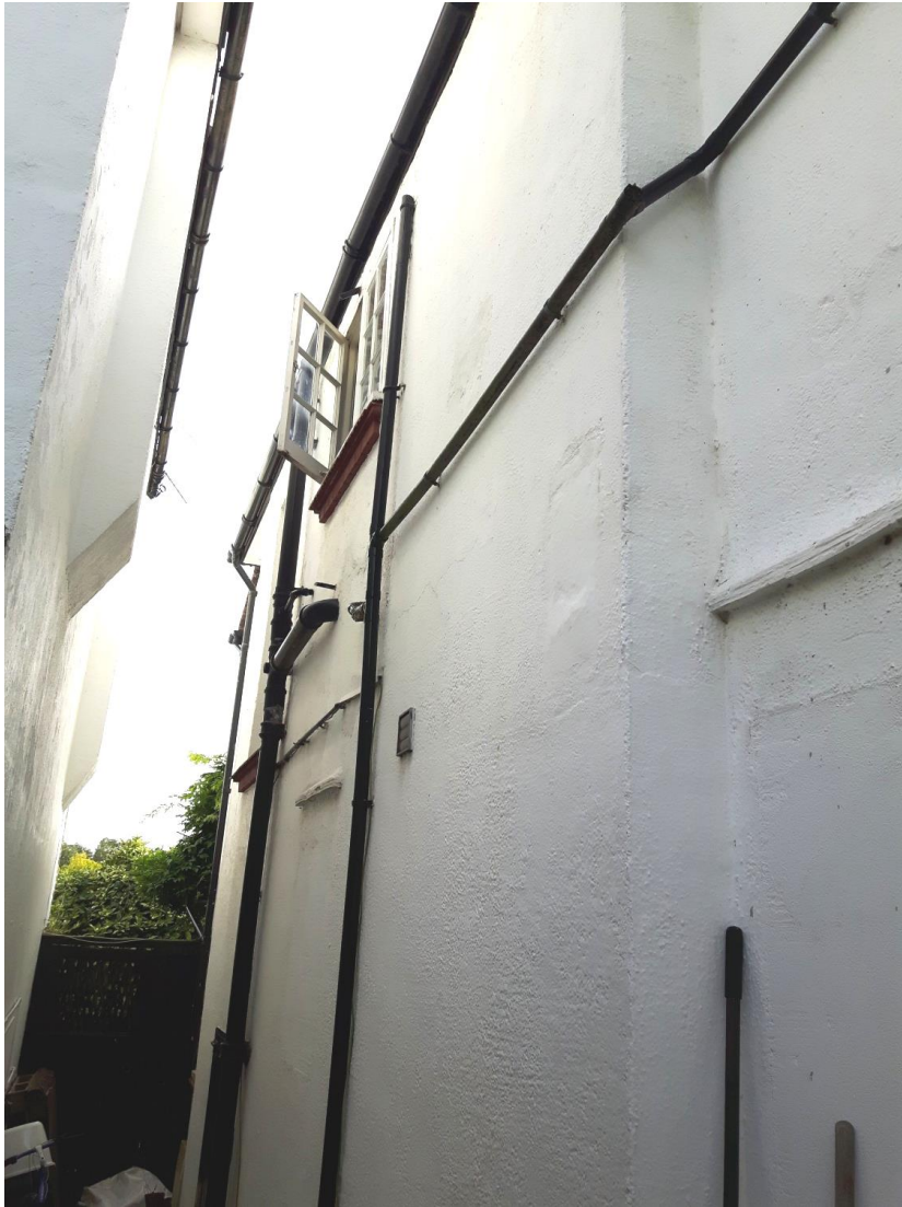
Fig. 5_ Side elevation towards No. 5 showing the blocked windows
