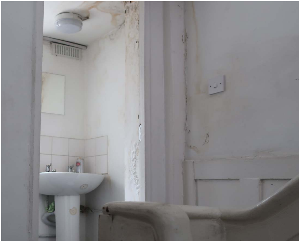
WC located off the first half level landing accessible from the internal staircase
