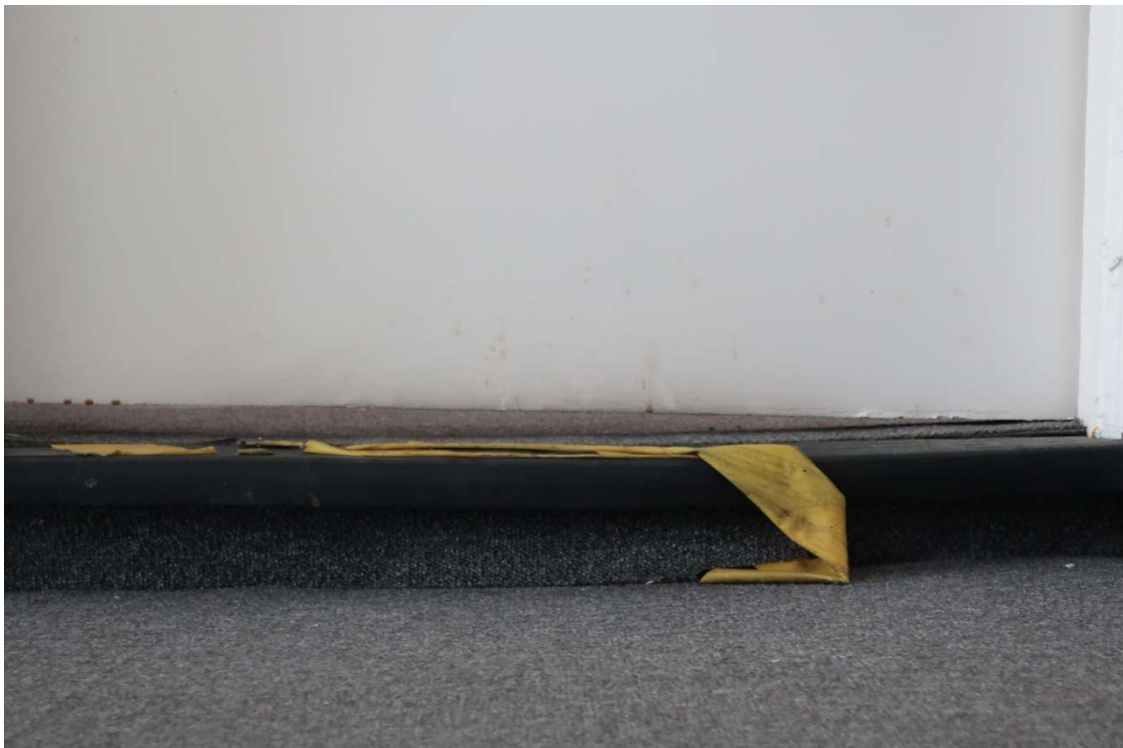
Door to second floor office from the second floor landing showing uneven flooring
