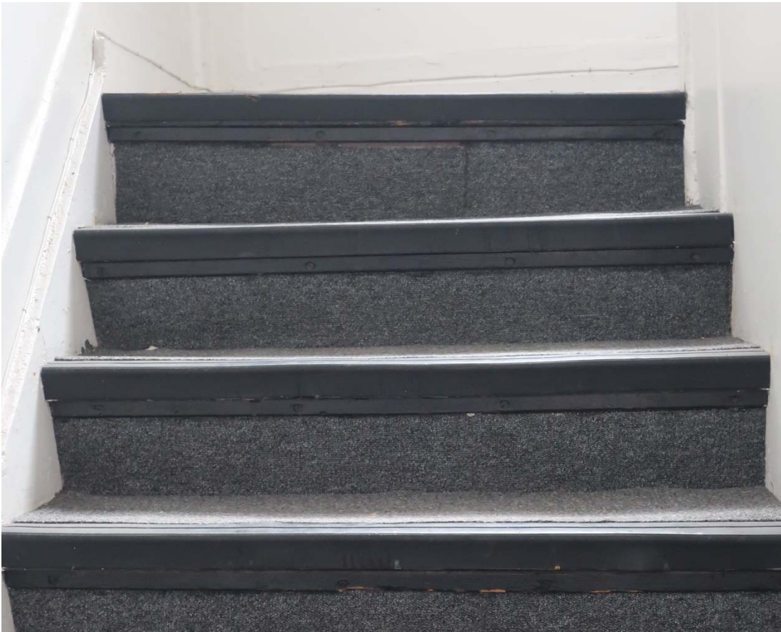
Uneven stair case and narrow foot treads to stairs from first floor landing up to the second floor landing
