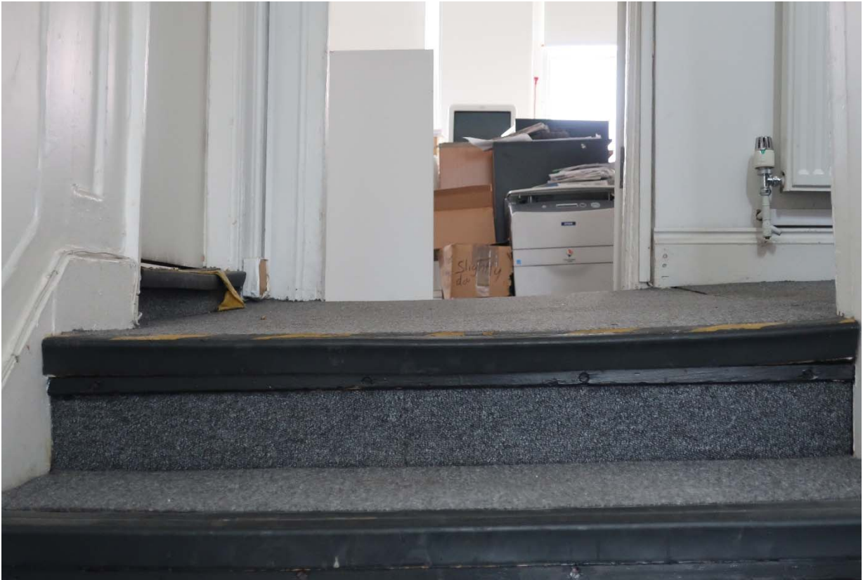
Stairs leading to second floor landing. Uneven stair case and severely uneven flooring to second floor landing
