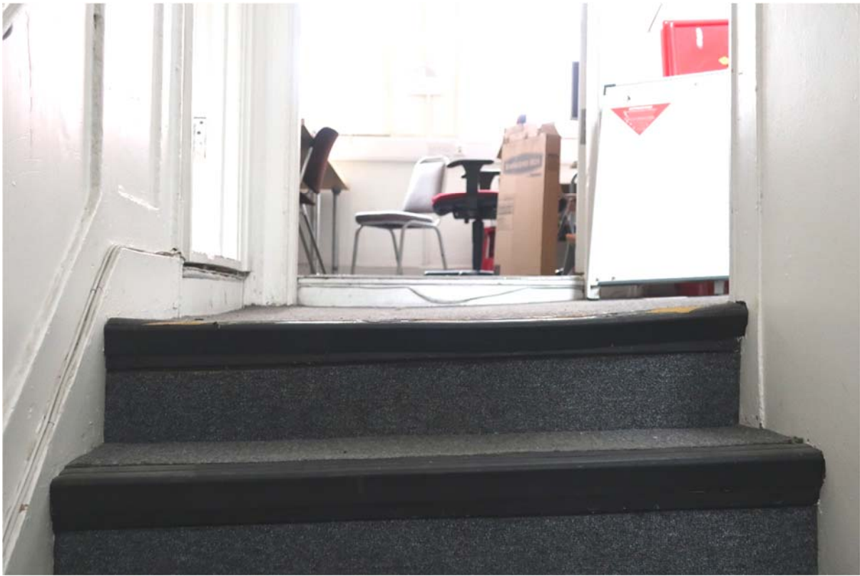
Stairs leading to the first floor landing. Uneven and narrow staircase leading to uneven flooring to landing
