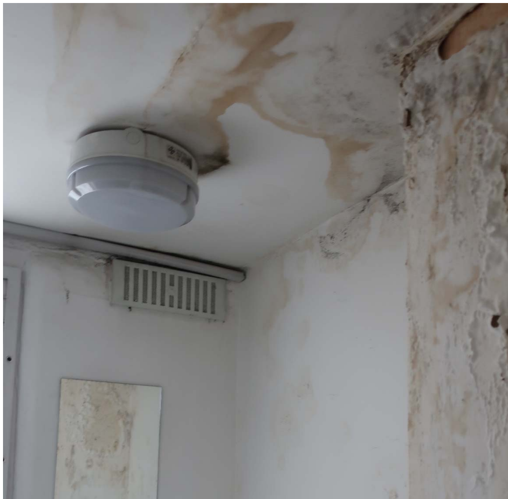
Water damage to the half level WC
