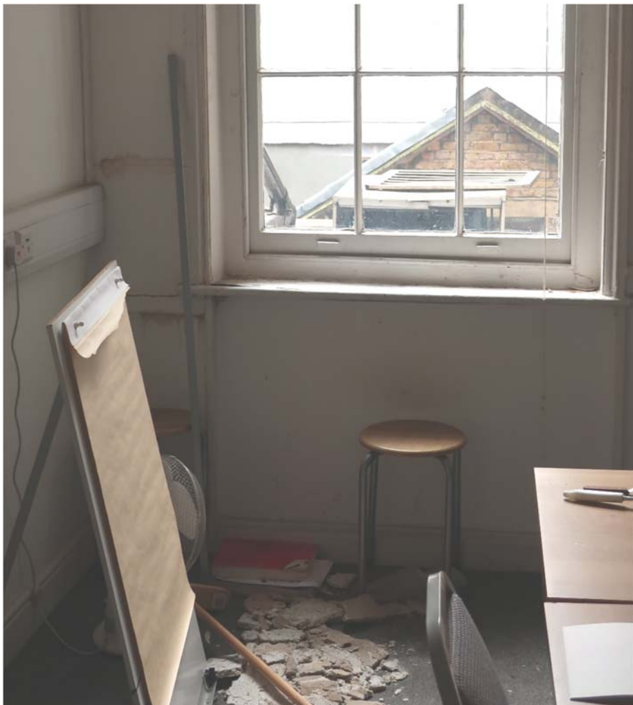
Water damage to first floor office
