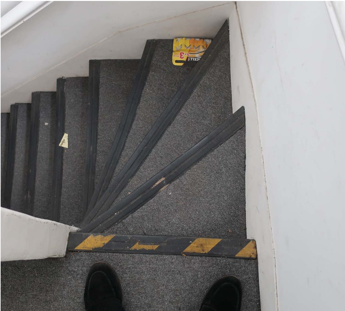
Uneven and narrow staircase foot treads from the third floor landing
