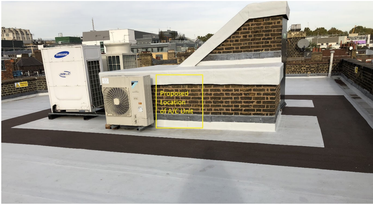
Photograph 2. Proposed Location of First Air Handling Unit
