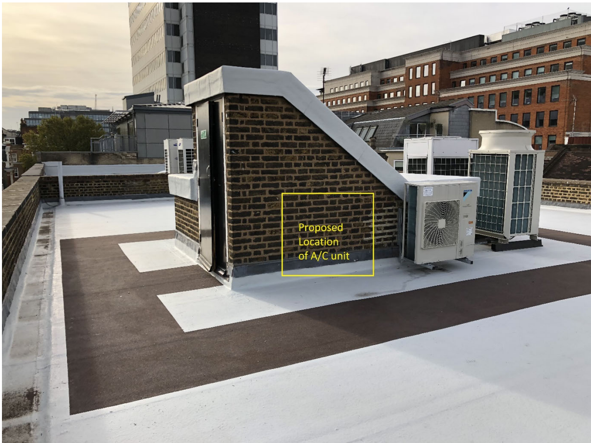
Photograph 3. Proposed Location of Second Air Handling Unit
