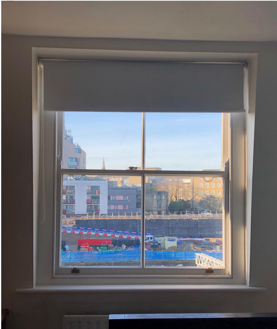
Figure 8: Internal view of window at third floor bedroom (Flat C)
