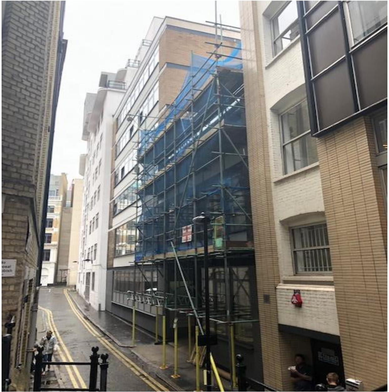
2. Rear elevation of application building (Onslow Street) as seen from Clerkenwell Road. The scaffolding relates to the construction of planning permission ref: 2016/4143/P for a first floor rear extension. The proposed extension would be built on top of this current construction.
