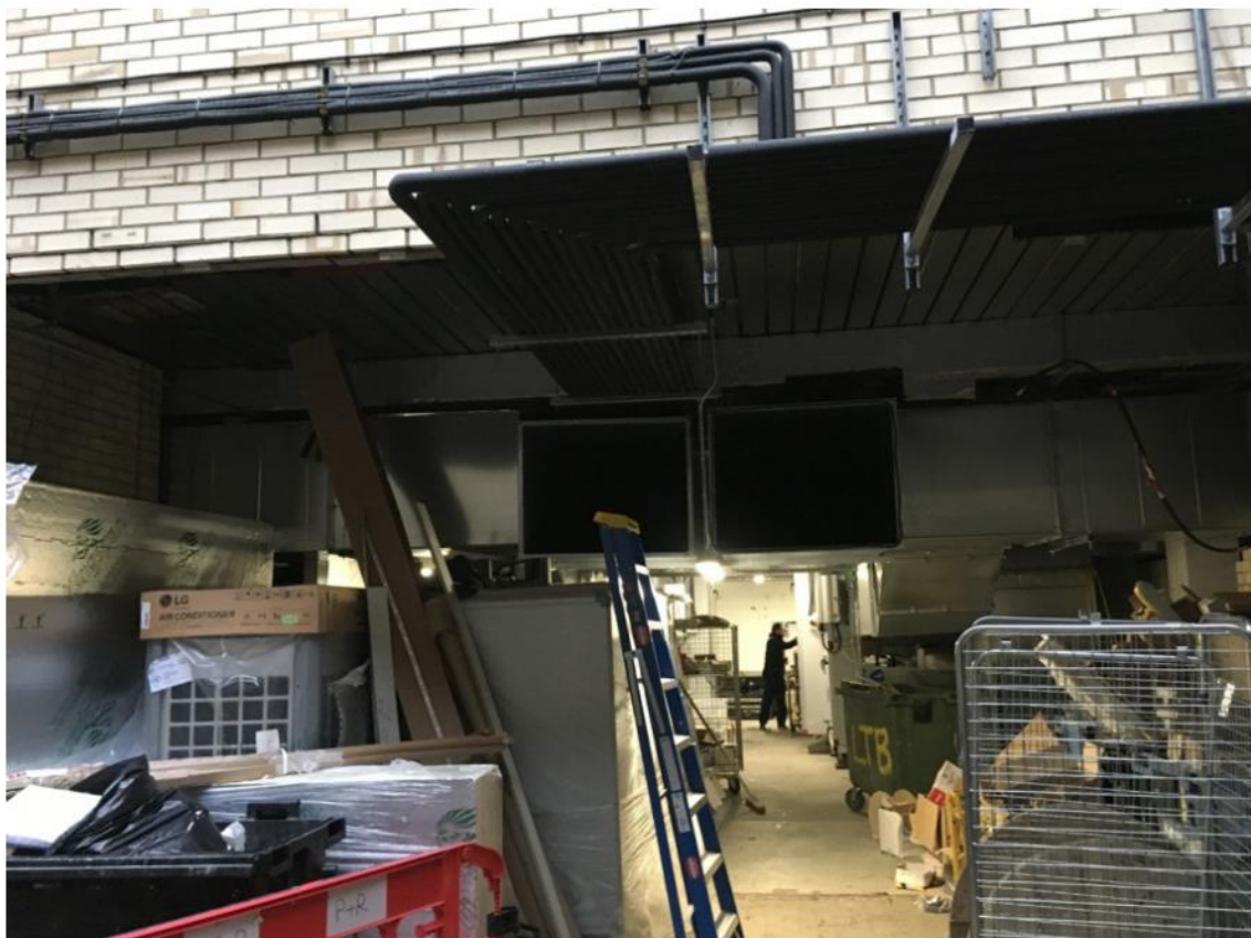
Image 2. Showing the ductwork and rear lightwell.
