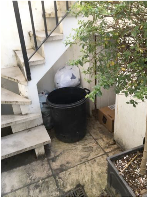
Front light well- existing stair and vault door, prior to removal of the stair
